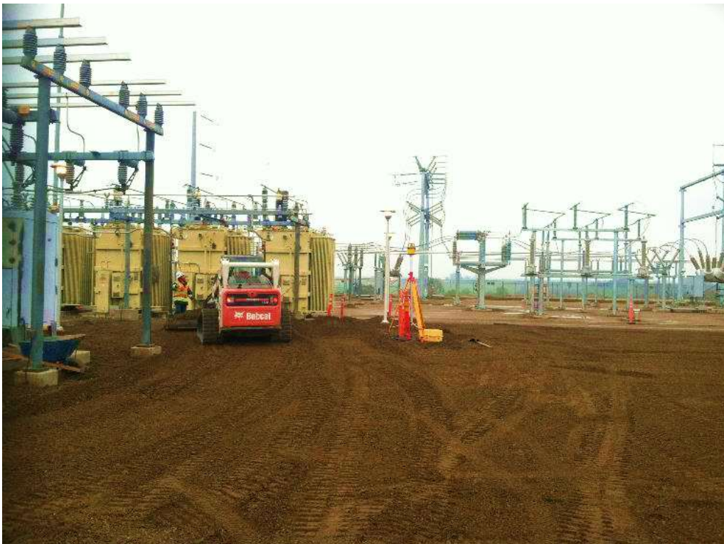
Figure 2 – Grading and paving work continued at Cressey Substation during the subject period. View east, 12/10/15.
