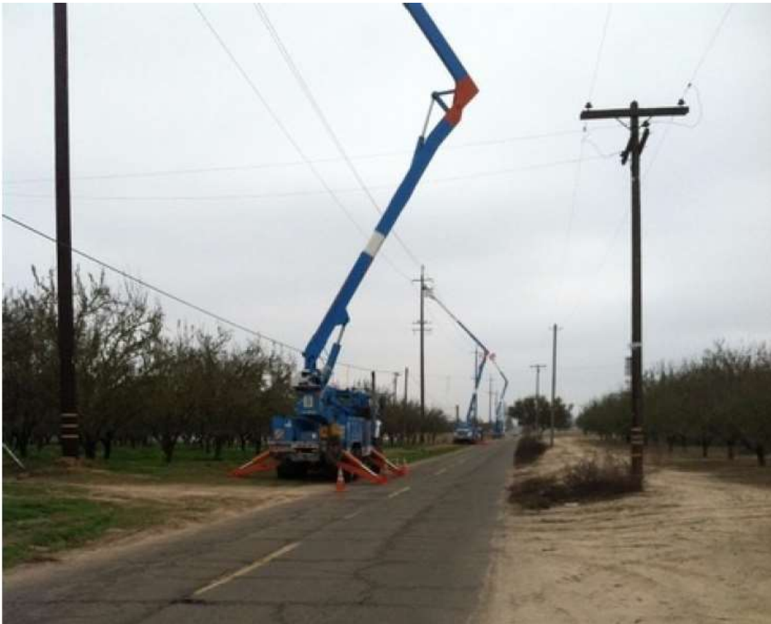
Figure 3 – Line work continued along Arena Way during the subject period. (Photo provided by PG&E).
