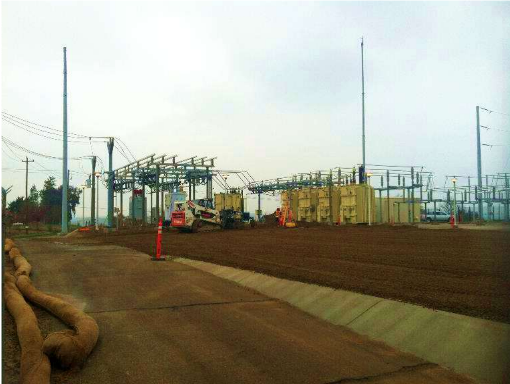
Figure 1 – Paving activities continued at the Cressey Substation during the subject period. View northeast, 12/10/15.
