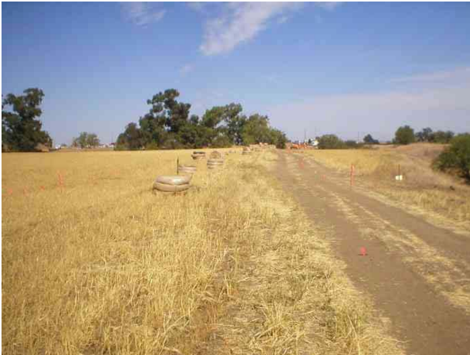
Figure 2 – The access road to the Delta Substation which had originally followed the dirt two track road has been shifted west by approximately 22 feet. Crews have installed lath and flagging which shows the new roadway boundaries. September 27, 2007.
