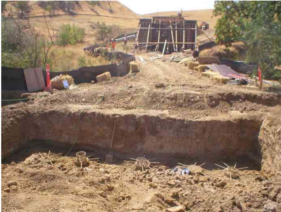
Figure 1 – Bridge foundation piers on the north side of Sand Creek have been completed. A form for the bridge riser was being constructed over the pier foundation on the south side of the creek. September 27, 2007.
