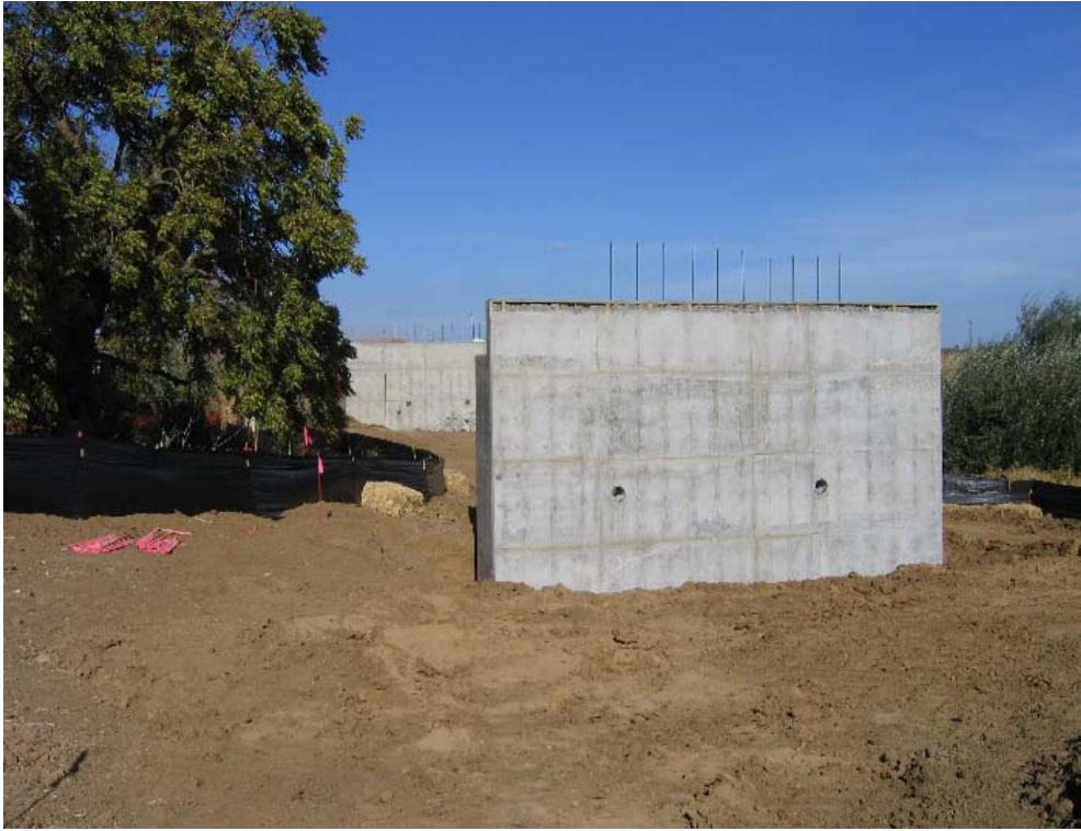
Figure 1 – View from south side of Sand Creek looking north at the two bridge foundations, October 10, 2007.
