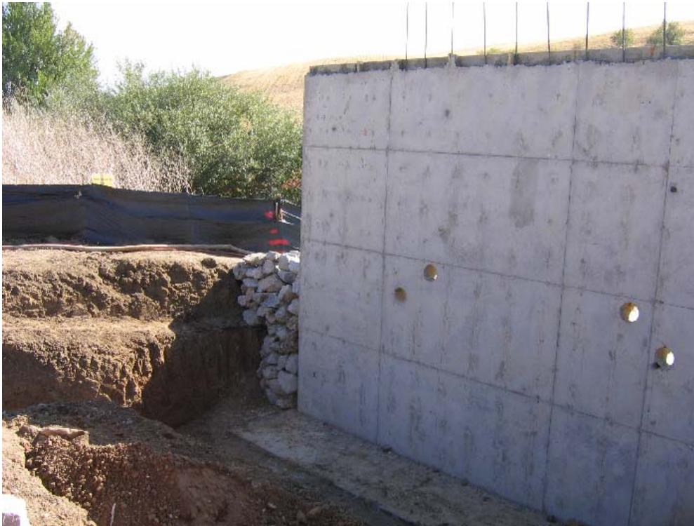
Figure 2 – North bridge foundation looking southeast showing foundation excavation and the beginning installation of riprap, October 10, 2007.
