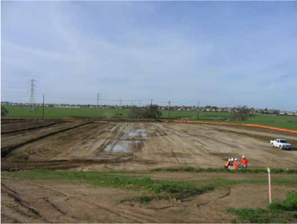
Figure 1 – PG&E Delta Substation site, February 26, 2008.
