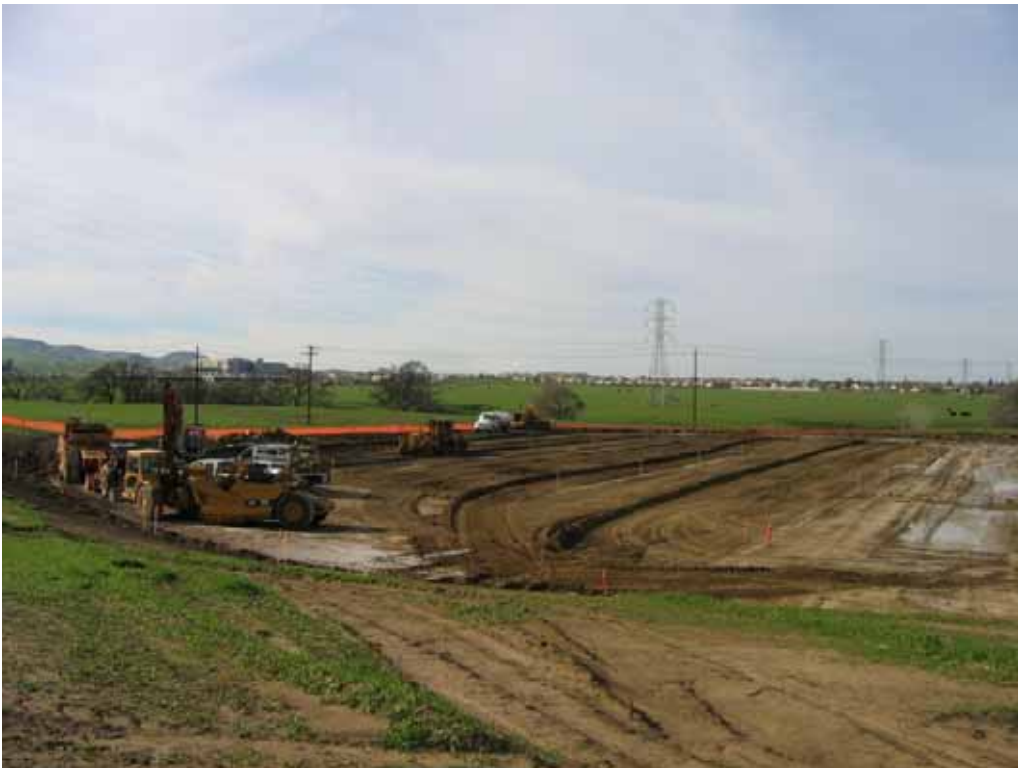
Figure 2 – Crews blading the western side of the substation site to dry it out, February 26, 2008.
