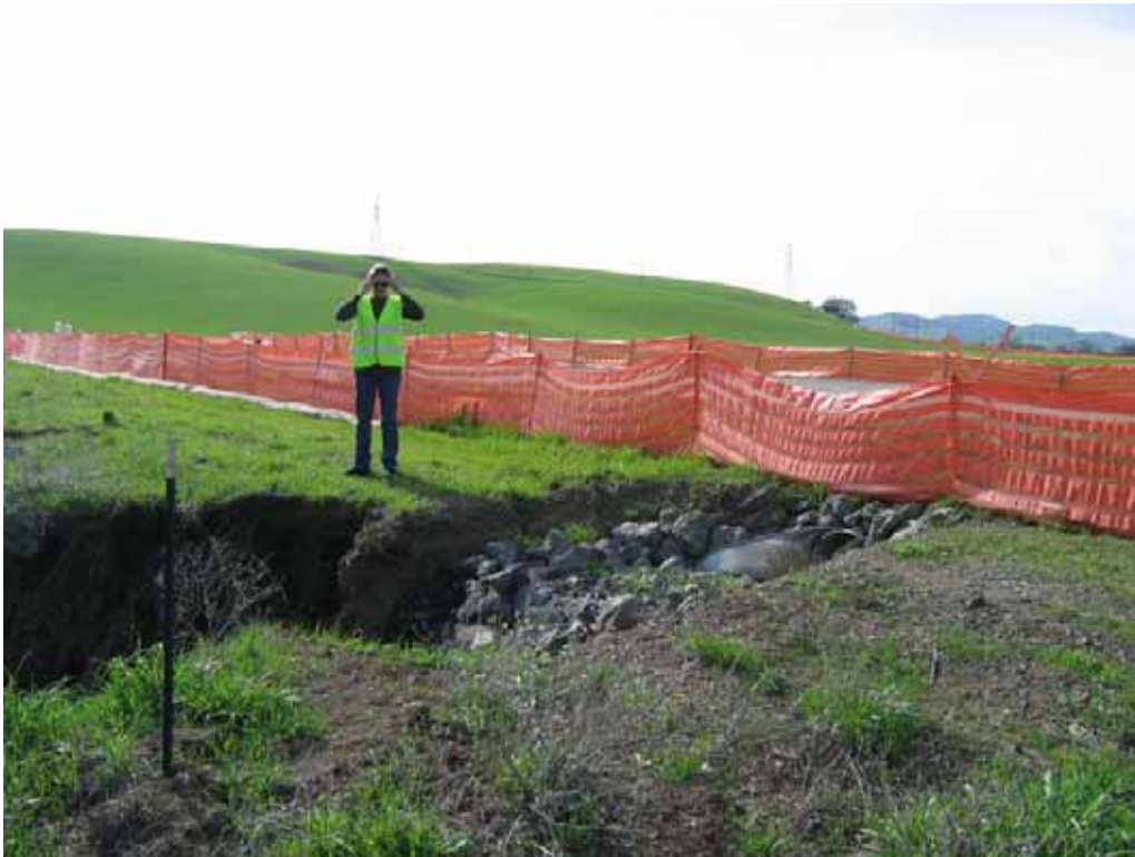
Figure 3 – Erosion problem at culvert outfall for Wetland #4 on south side of access road, February 26, 2008.
