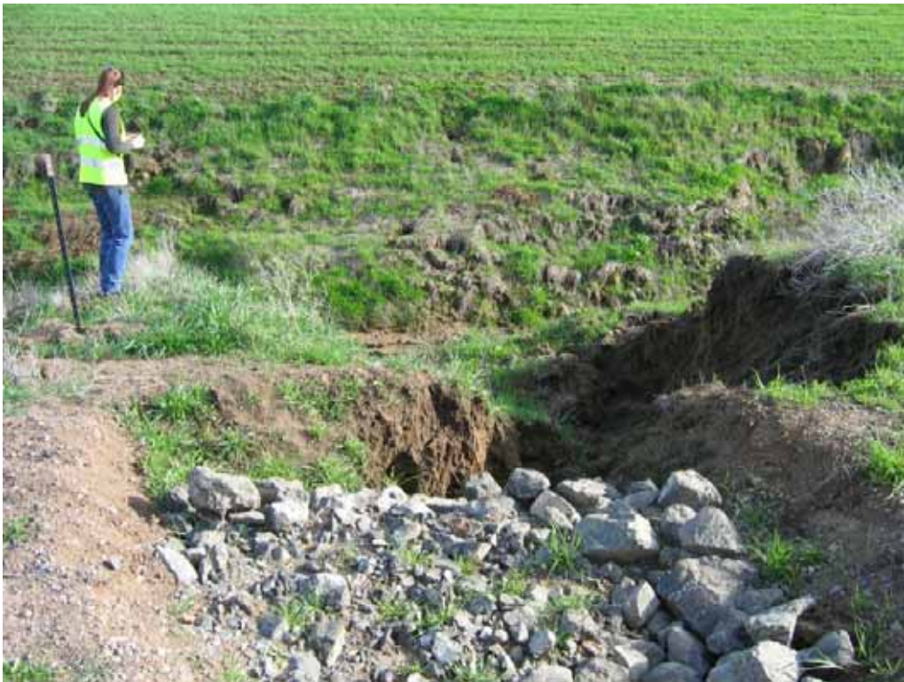
Figure 4 – Erosion problem at culvert outfall for Wetland #4 on south side of access road, February 26, 2008.
