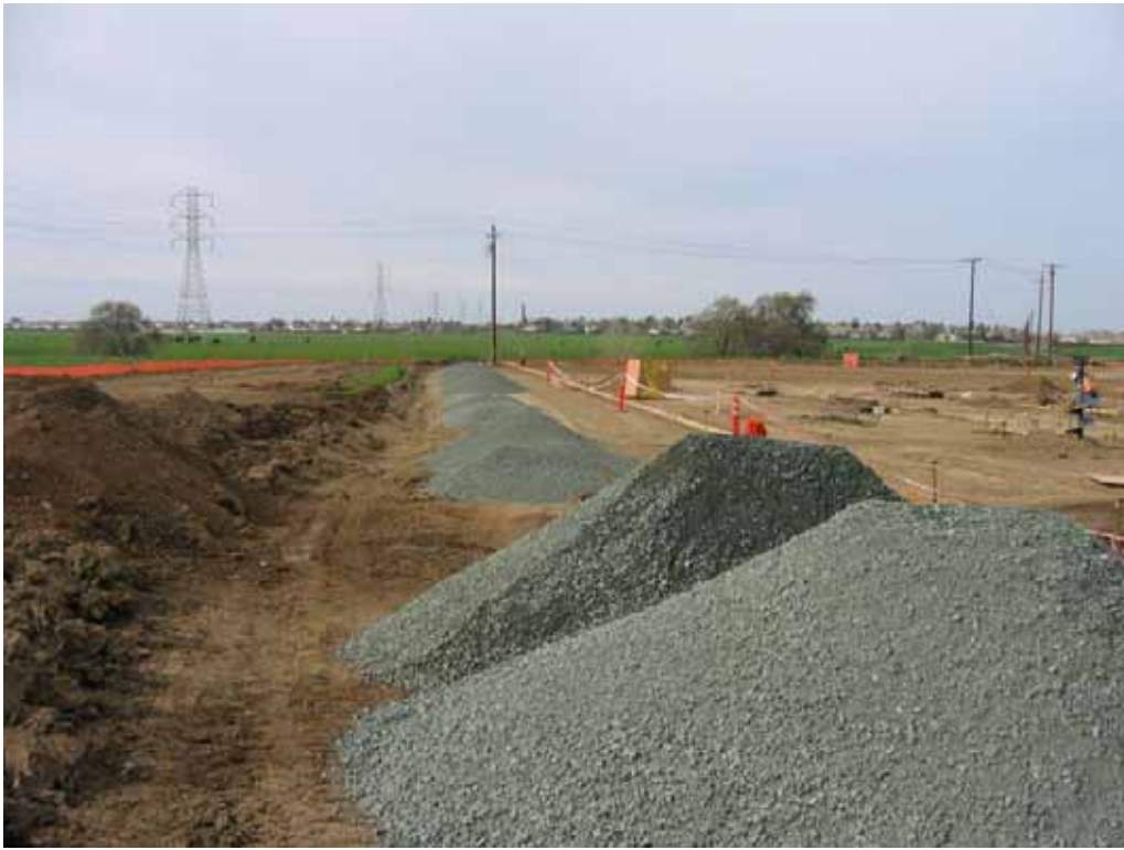
Figure 3 – Area where office trailers will be placed on the west side of the substation site, March 7, 2008.
