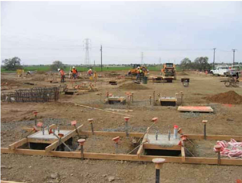
Figure 2 – Crews constructing foundation forms and pouring concrete foundations at substation site, March 7, 2008.
