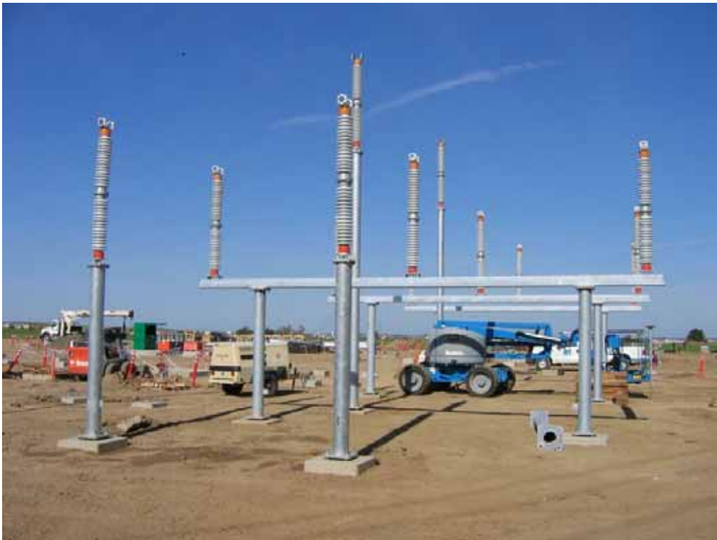
Figure 2 – Buss support structures partially installed in southwest corner of substation site, March 27, 2008.
