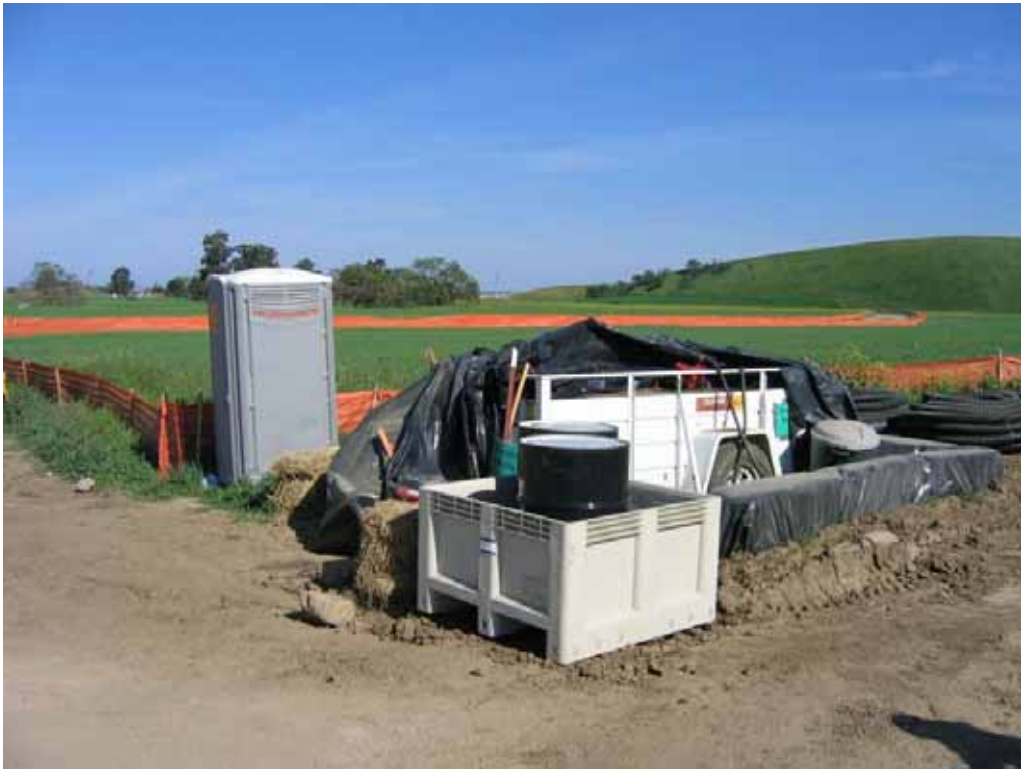
Figure 5 – New fuel container with two 55-gallon drums, March 27, 2008.
