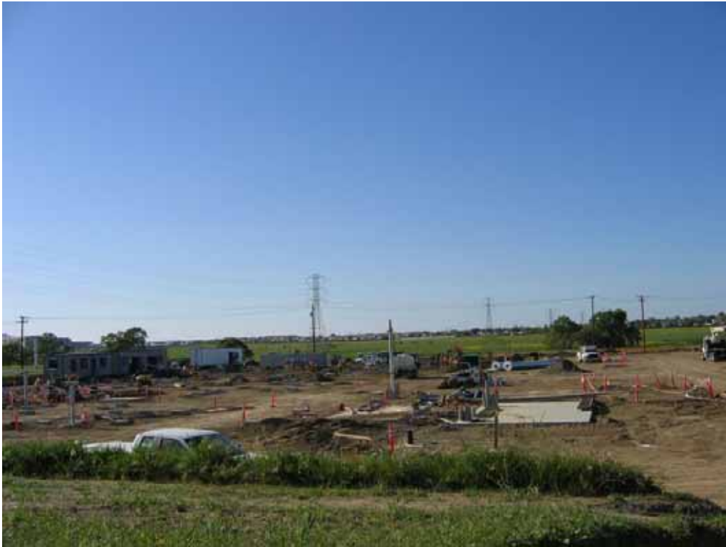
Figure 1 – View of substation site looking northwest, March 27, 2008.
