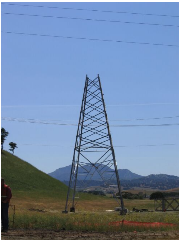
Figure 4 – Tower for the 230 kV loop, April 30, 2008.
