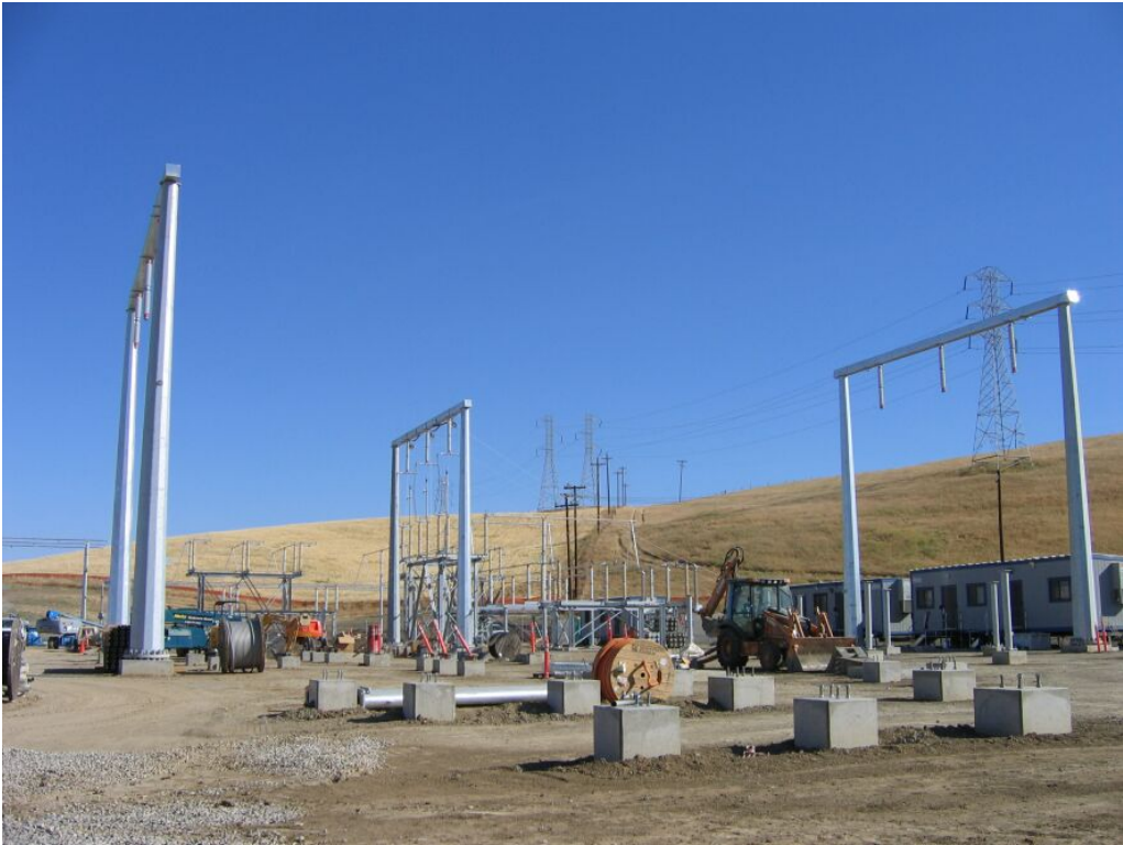
Figure 1 – Buswork structures at substation site, May 16, 2008.
