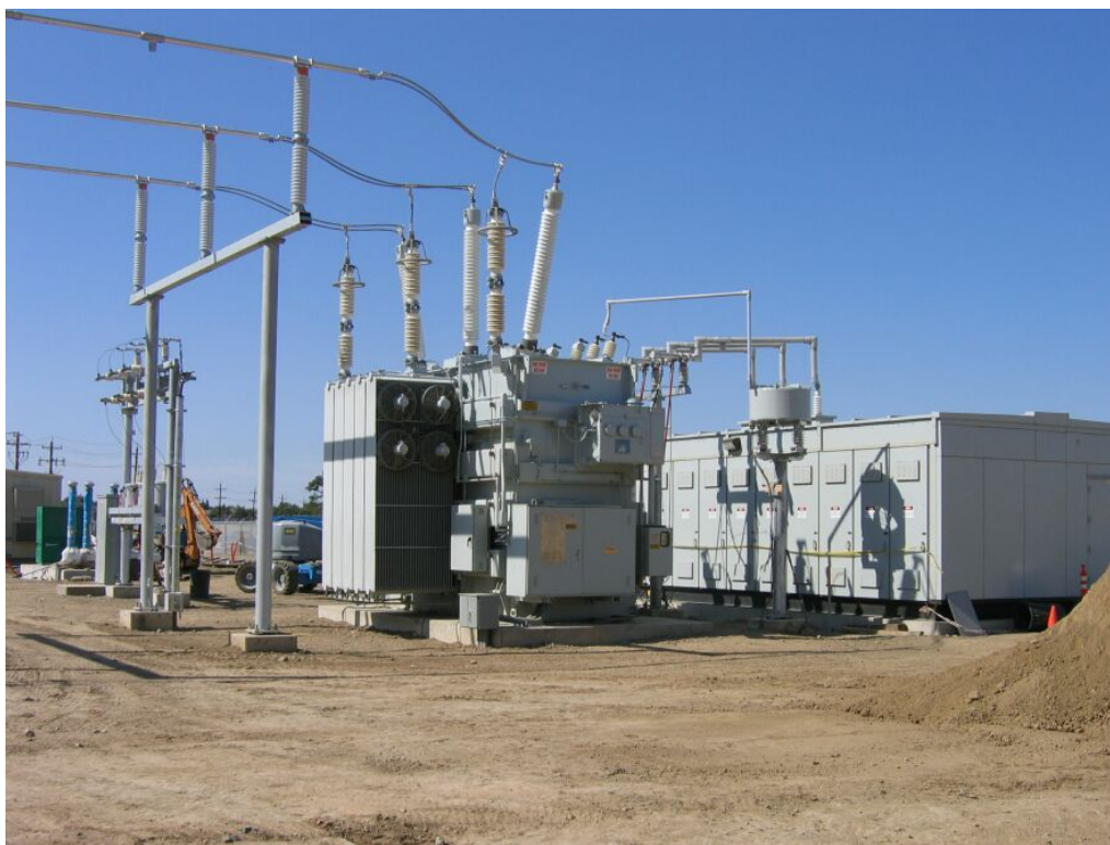
Figure 1 – Transformer and switchgear room at substation site, May 29, 2008.
