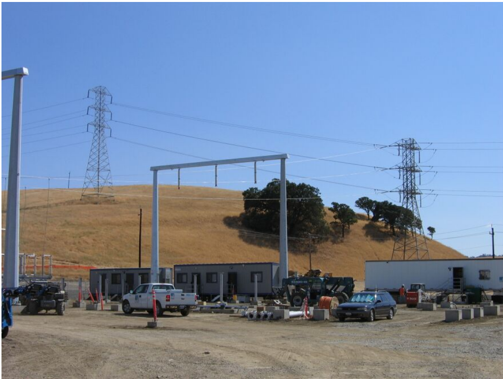
Figure 3 – New tower with lines connecting into substation, May 29, 2008.
