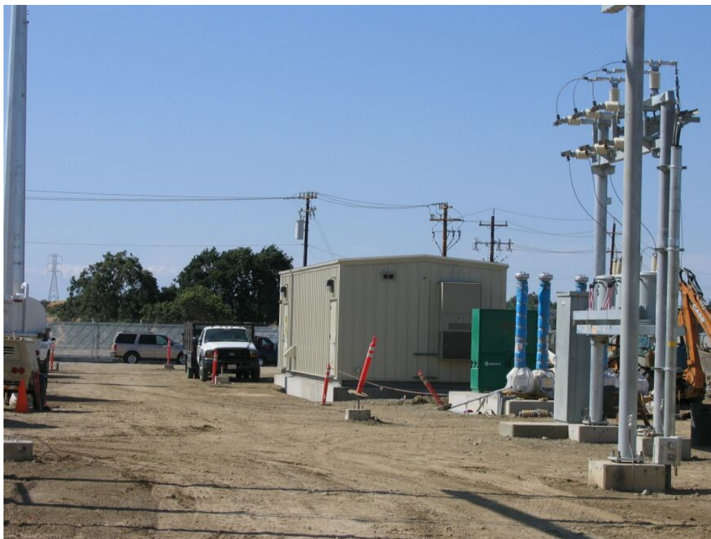
Figure 2 – MPAC building at substation site, May 29, 2008.
