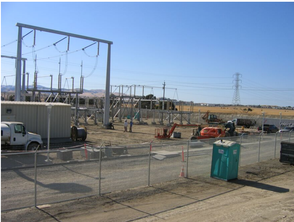
Figure 2 – View of substation site looking northwest, September 18, 2008.
