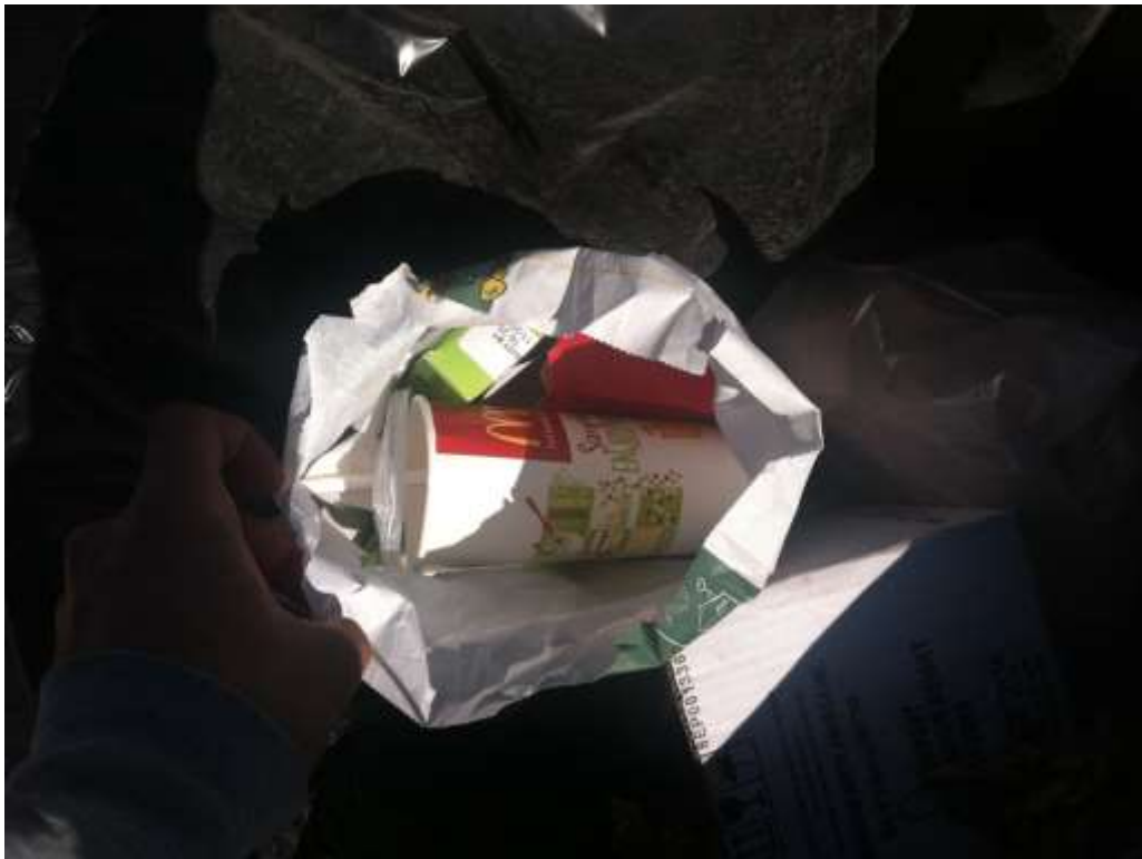
Figure 5 – Food trash left onsite uncovered after work hours. November 21, 2014.
