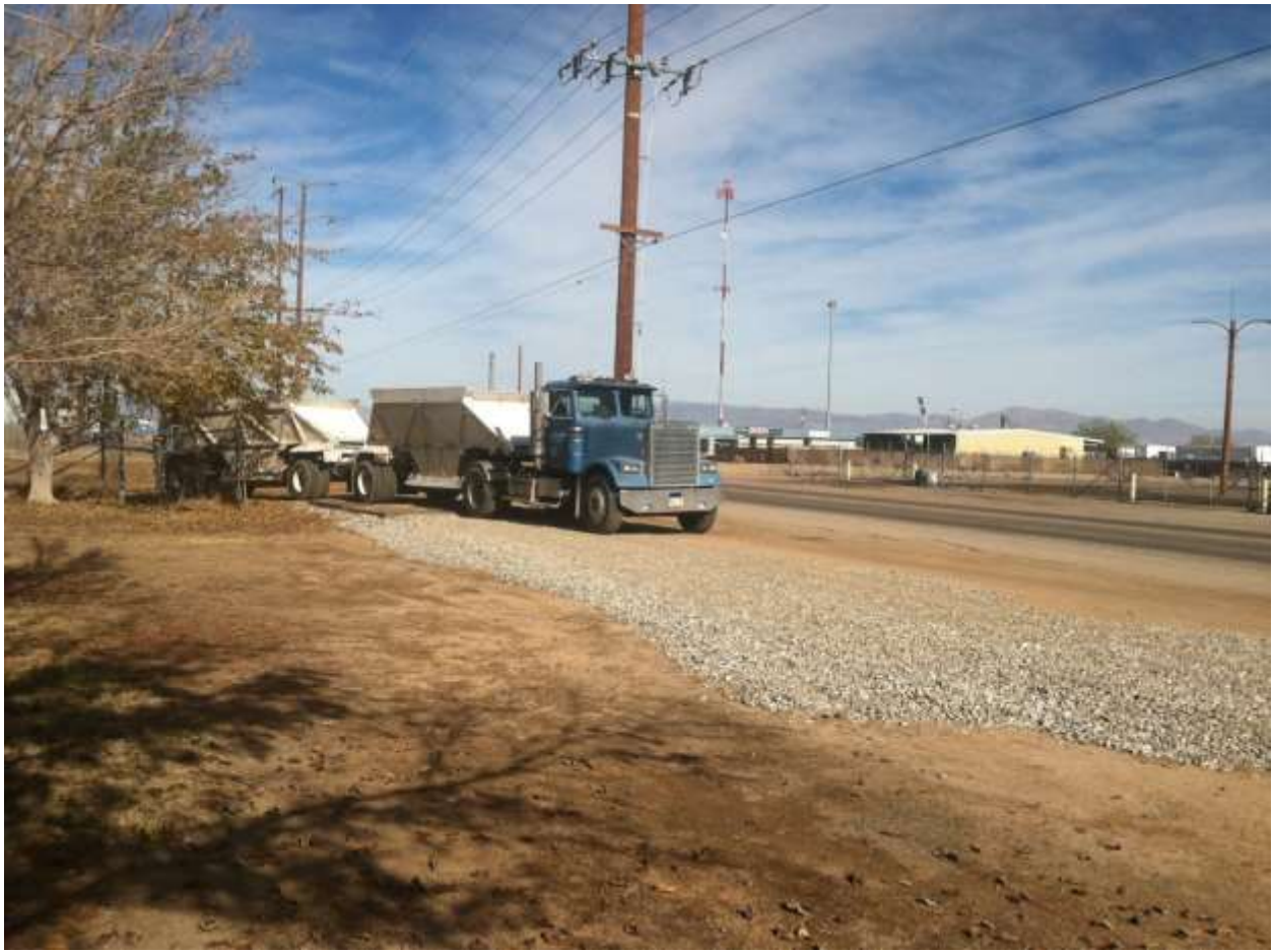
Figure 5 – A soil delivery truck exits the Project area using a rumble strip and gravel apron. View northeast, December 9, 2014.
