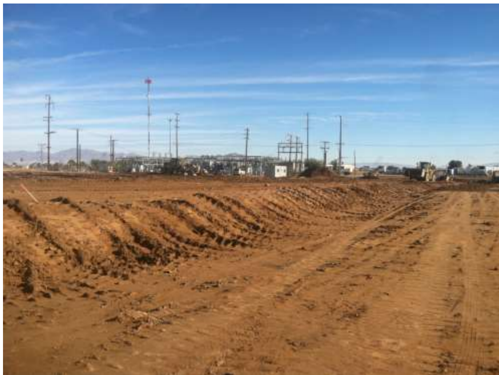
Figure 2 – Grading continued. Leveling and compacting of substation expansion area pad is progressing. View northeast, December 9, 2014.
