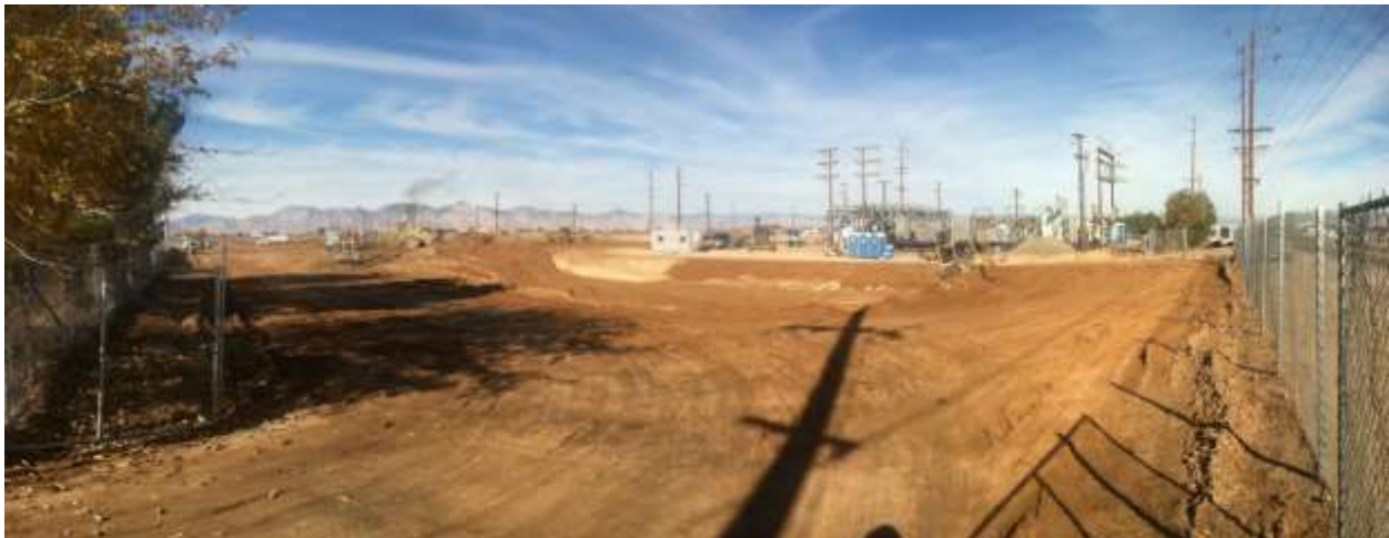
Figures 3&4 – Panoramic view of detention basin grading progress, from southeast corner of site. Week #3 12/4/14 above, Week #4 12/9/14 below, view northwest.
