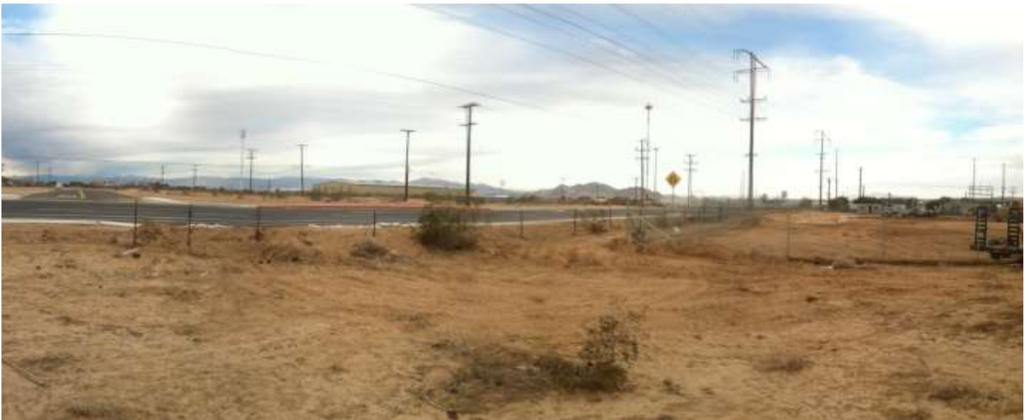
Figures 5&6– Soil pile and disturbance are seen just outside the northwest corner of the Project work area. Week #4 (12/9/14) before removal and compaction (above), and Week #5 (12/15/14) after removal and compaction (below), view northeast.
