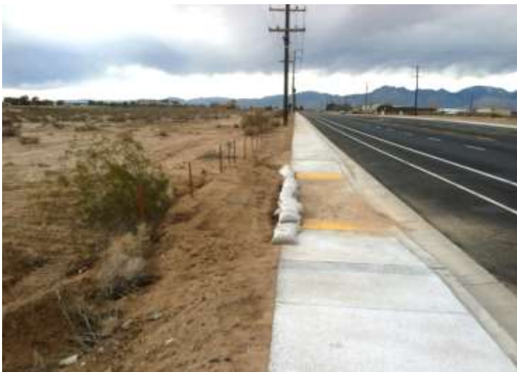
Figures 7, 8 &9– Soil pile was removed/compacted, along Ridgecrest Boulevard. 12/4/14 top (prior to soil addition), 12/9/14 middle (after soil addition), 12/15/14 bottom (after soil removal/compaction), view west.
