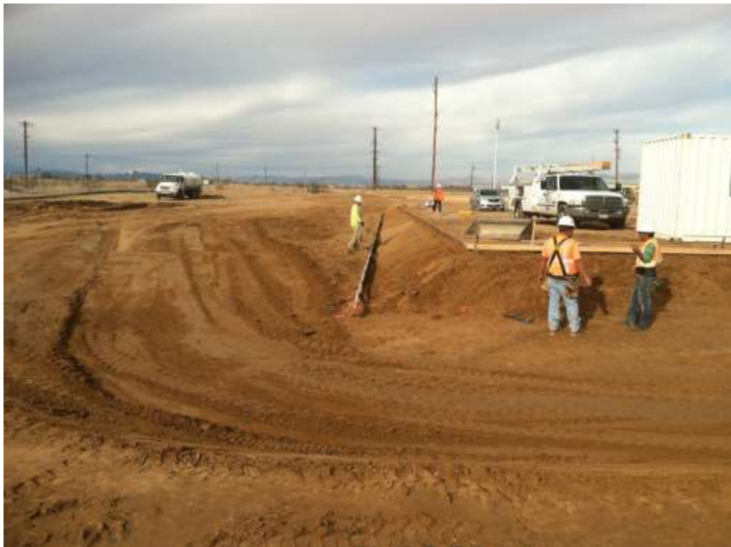
Figure 2 – Grading continued. Leveling and compaction of the substation expansion area pad is progressing. View north, December 15, 2014.
