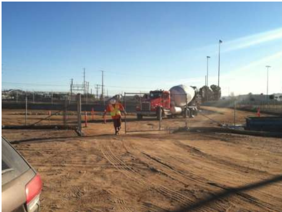
Figure 7 – A concrete truck leaves the work area through the recently approved access per MPC #1. View eastward, January 8, 2015.
