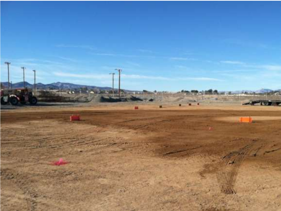
Figure 1 – Surveyor markers have been installed on the Substation pad. View southeast, January 8, 2015.
