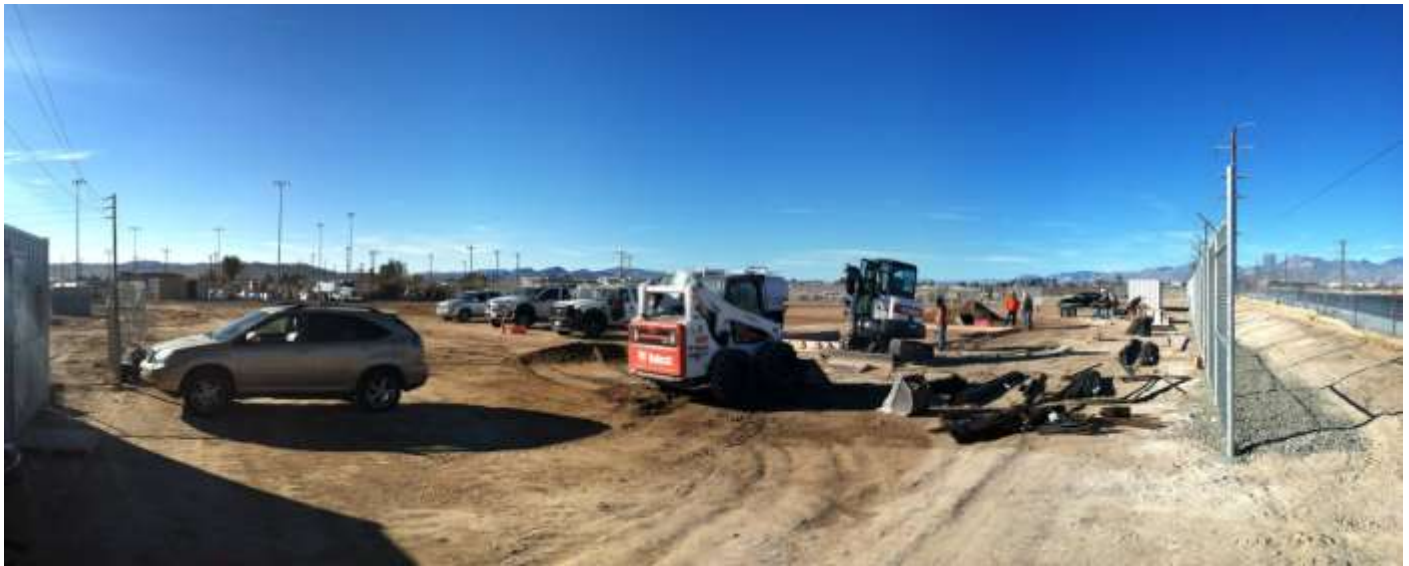
Figure 4 – Installation of a MEER building began during the subject period.. View from the northeast corner of the substation pad, facing southwest, January 8, 2015.
