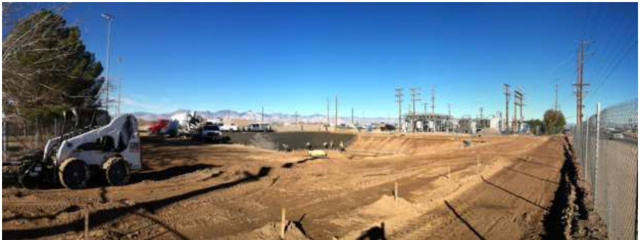
Figure 5 – Panoramic view of detention basin grading progress, from southeast corner of site. 12/15/14 above, 12/23/14 middle, 01/08/15 below, view northwest.
