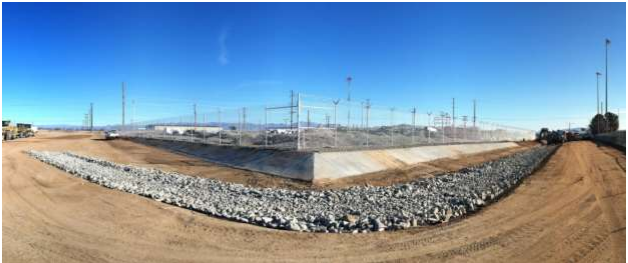
Figure 3 – Fence installation continued. Storm water devices were installed. 12/23/14 above, 01/08/15 below, view northeast.
