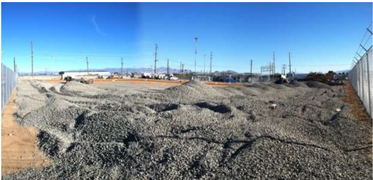
Figure 2 – Gravel is positioned along the south edge of the substation pad. View from the southwest corner of the substation pad facing northeast, January 8, 2015.
