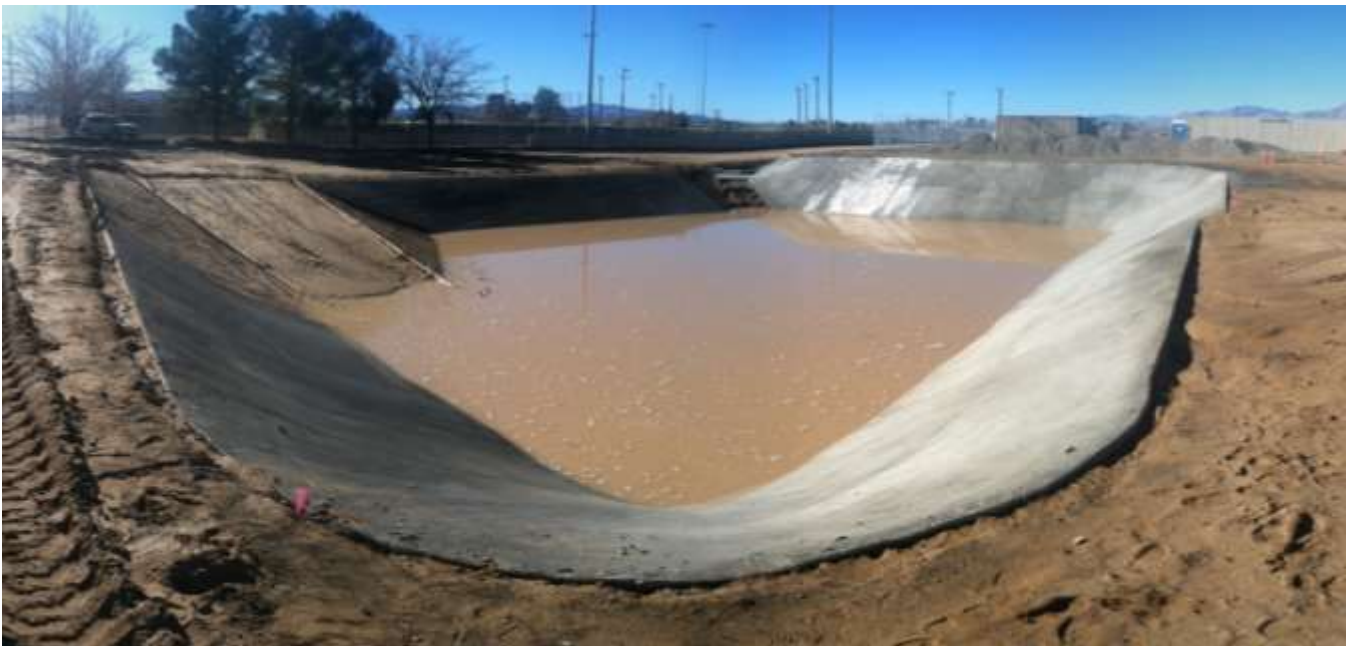
Figure 7 – Installation of the detention basin continued. Weekend rains deposited some water here. View southwest, 01/08/15 above and 01/13/15 below.
