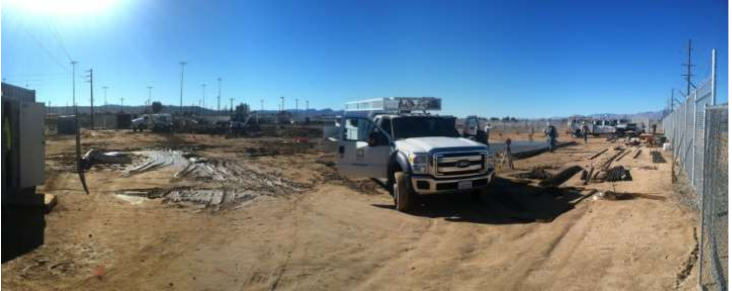
Figure 5 – Installation of a MEER building continued during the subject period. View from the northeast corner of the substation pad. View southwest, 01/08/15 above and 01/13/15 below.
