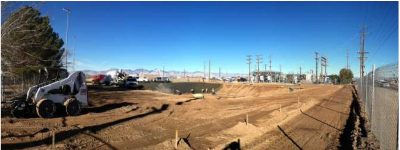
Figure 6 – Panoramic view of detention basin grading progress, from southeast corner of site. View northwest, 12/23/14 above, 01/08/15 middle, and 01/13/15 below.
