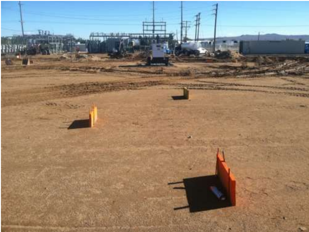
Figure 1 – Surveyor markers have been installed on the substation pad in preparation of structure installation. View east, January 13, 2015.
