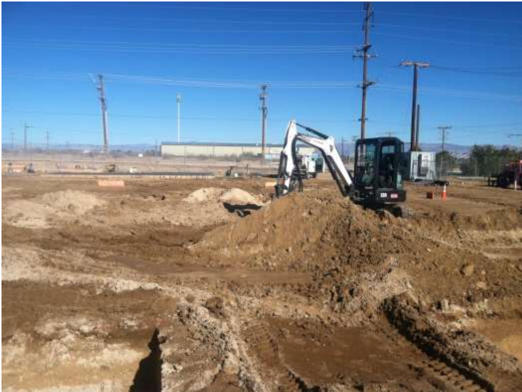
Figure 3 – Trenching occurred at the substation pad during the subject period. View northeast, January 13, 2015.
