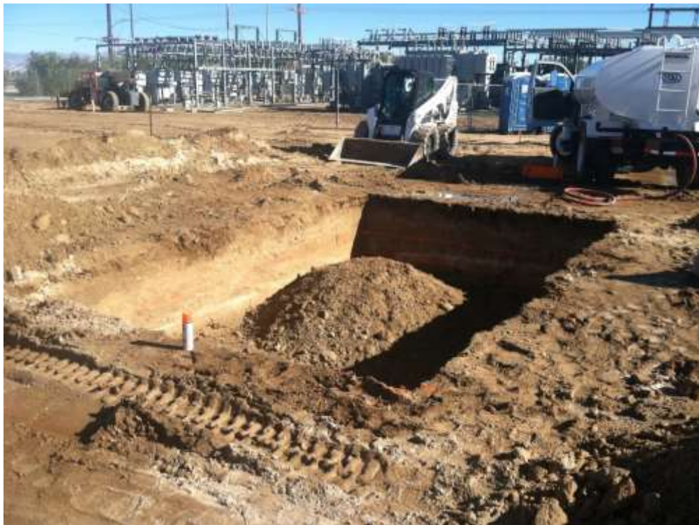
Figure 2 – Trenching occurred at the substation pad during the subject period. View northeast, January 13, 2015.
