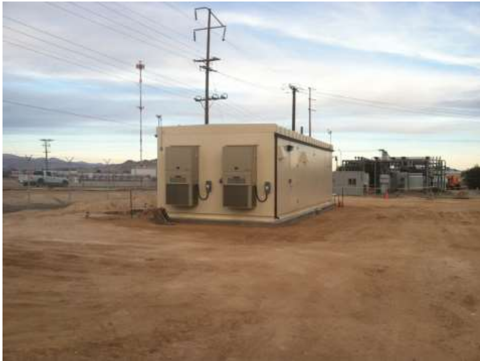
Figure 3 – Installation of the MEER building occurred during the subject period. View northeast, January 22, 2015.
