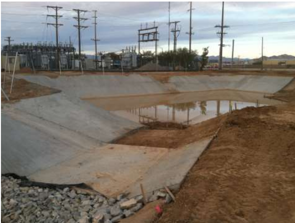
Figure 4 – Pooled water has delayed completion of the site's detention basin. View northeast, January 22, 2015.
