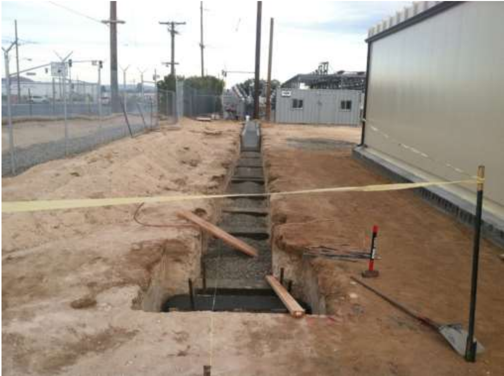
Figure 7 – A trench was equipped with escape ramps to help prevent animal entrapment. View east, January 22, 2015.
