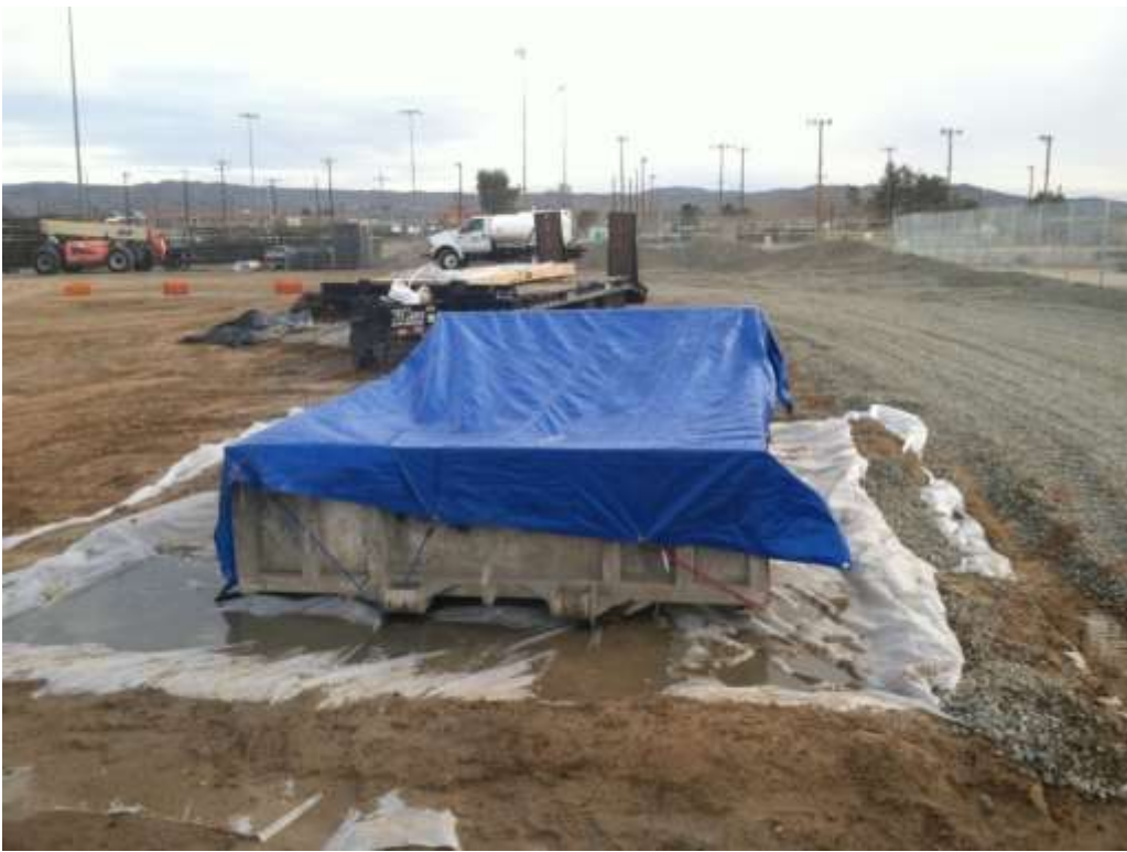
Figure 6 – Concrete washout is properly contained at the end of the work day. View south, January 22, 2015.
