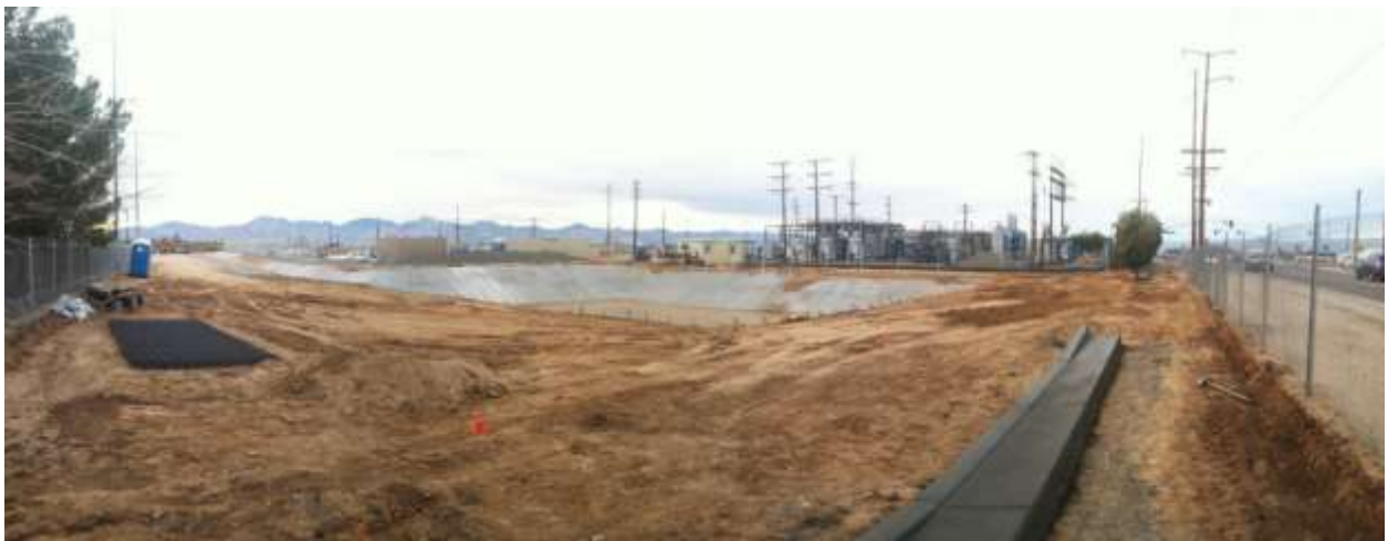
Figure 5 – Panoramic view of detention basin grading progress, from southeast corner of site. View northwest, 01/08/15 above, 01/13/14 middle, and 01/22/14 below.
