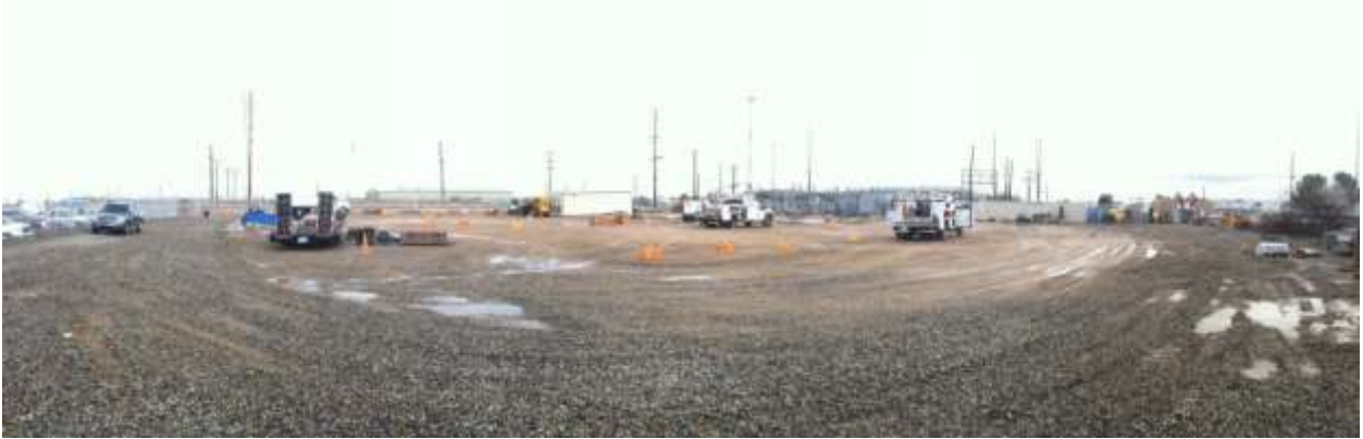
Figure 1 – Gravel and materials continue to be stored on the substation pad. View northeast, January 27, 2015.
