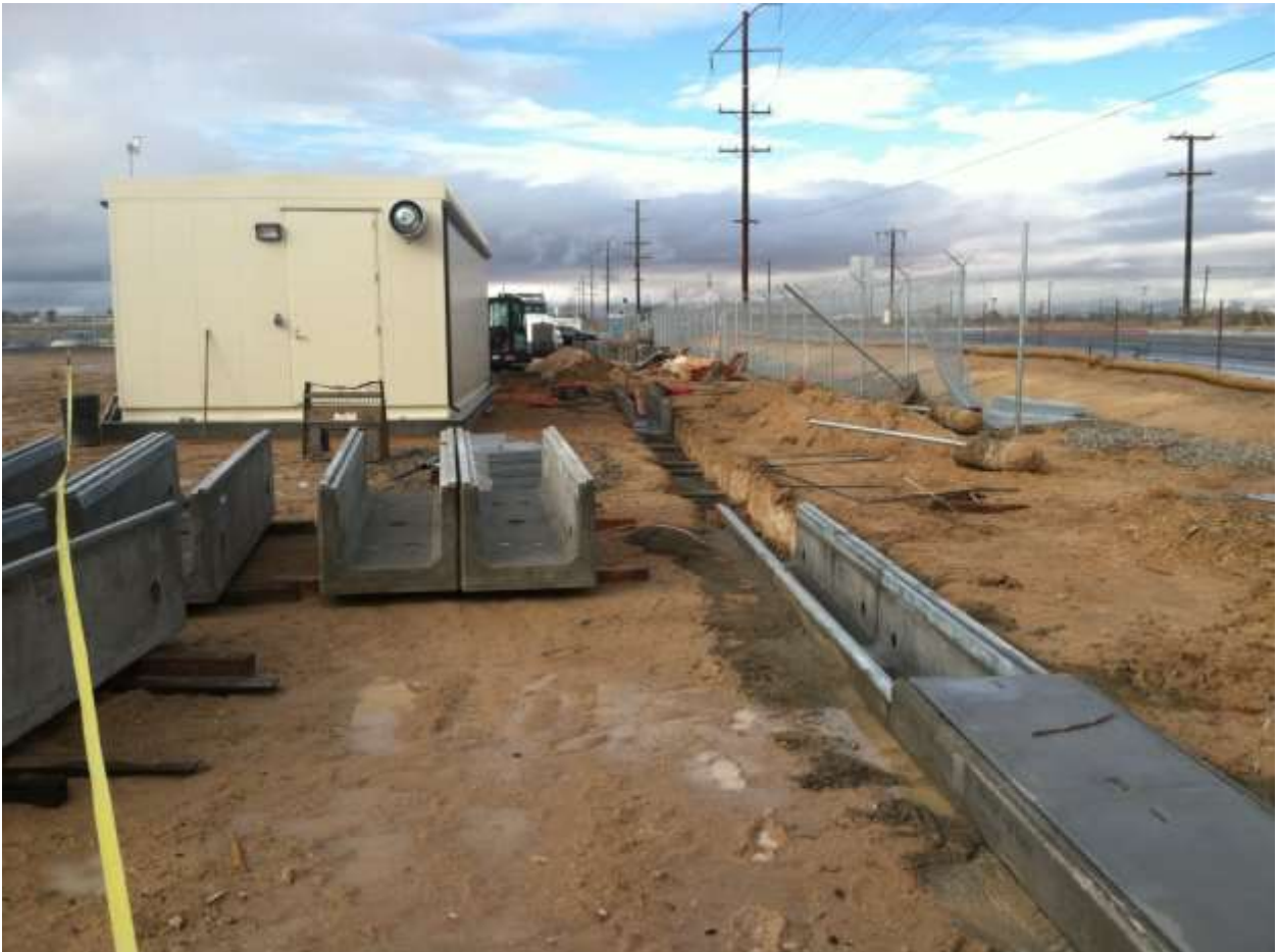
Figure 2 – Installation of the MEER building and associated wiring occurred during the subject period. View west, January 27, 2015.
