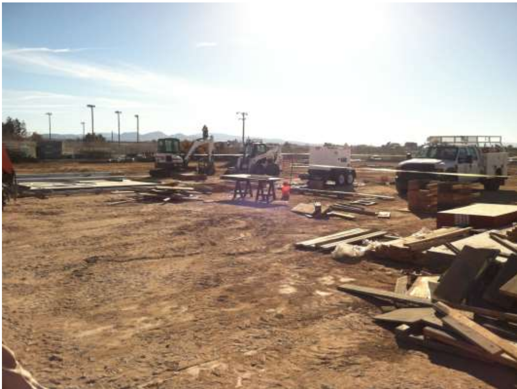
Figure 3 – Augering, trenching, and foundation installation continued in the substation expansion area. View southwest, 02/19/15.
