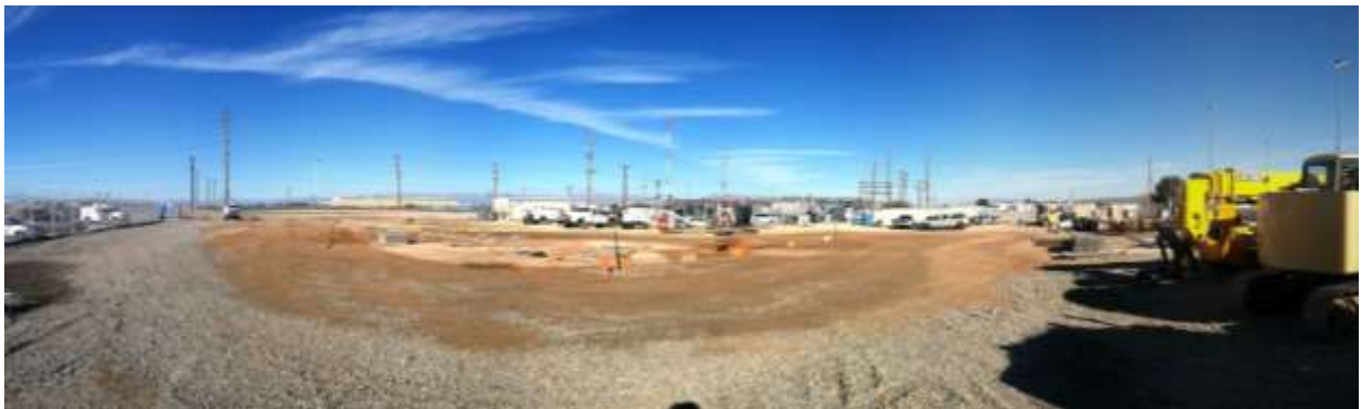
Figure 1 – Gravel and materials continue to be stored on the substation pad. View northeast, 01/27/15 above, 02/06/15 middle, 02/19/15 below.
