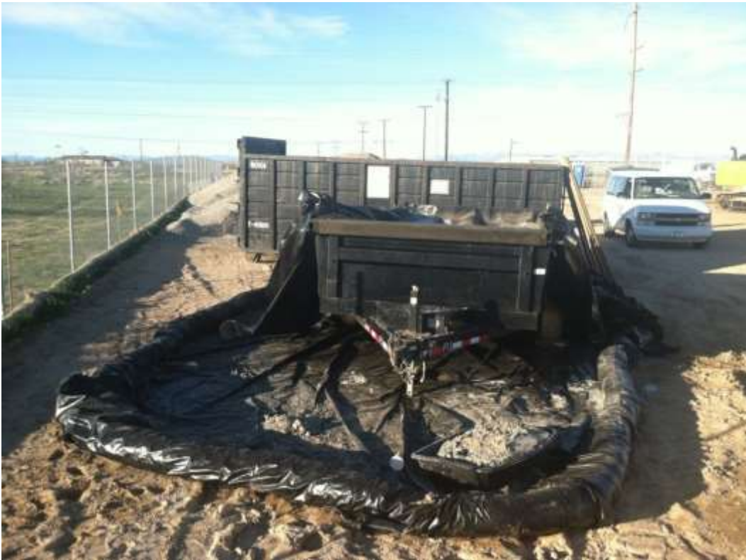
Figure 4 – Concrete washout is secured at the end of the day. View north, 02/26/15.
