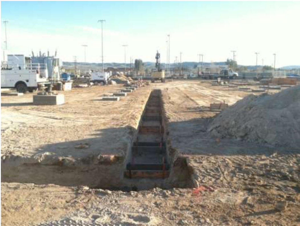
Figure 3 – Augering, trenching, and foundation installation continued in the substation expansion area. View south, 02/26/15.
