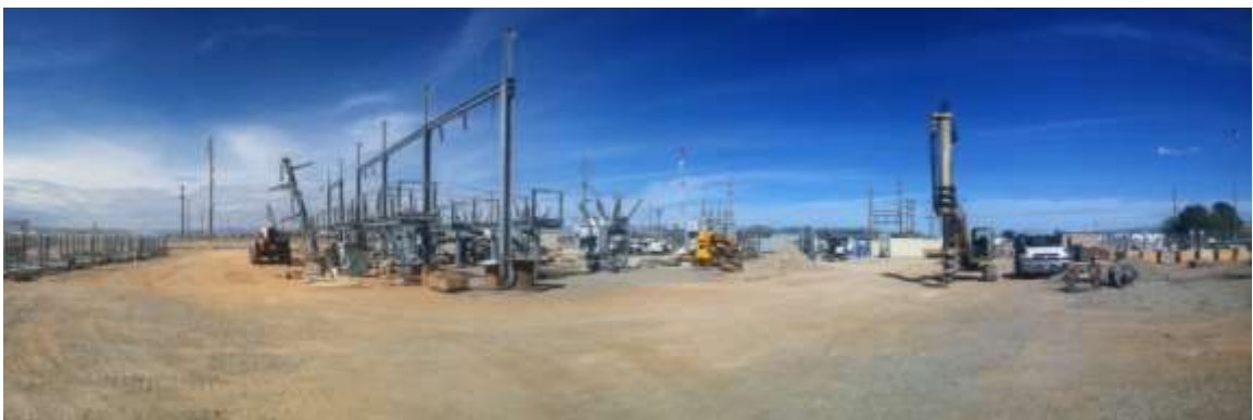
Figure 1 – Installation of the substation pad continued during the subject period. View northeast, from top: 01/27/15, 02/06/15, 03/17/15 and 03/24/15.
