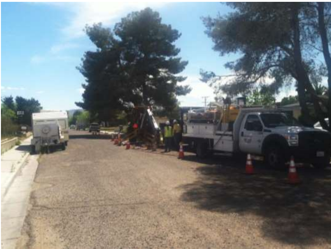
Figure 5 – Boring work for telecom lines continued during the subject period. View south, 03/24/15.
