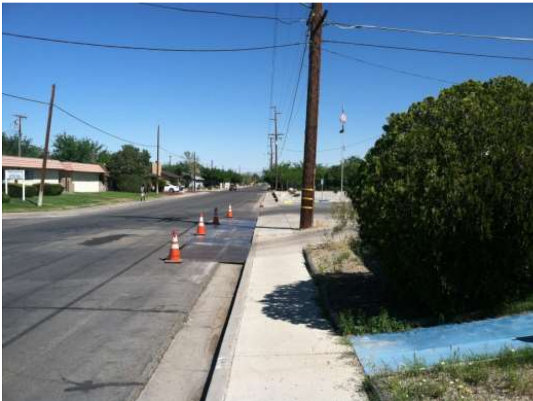
Figure 5 – Boring work for telecom lines continued during the subject period. Steel plates are seen at the future location of the telecom line riser pole along East Church Avenue. View east, 03/30/15.
