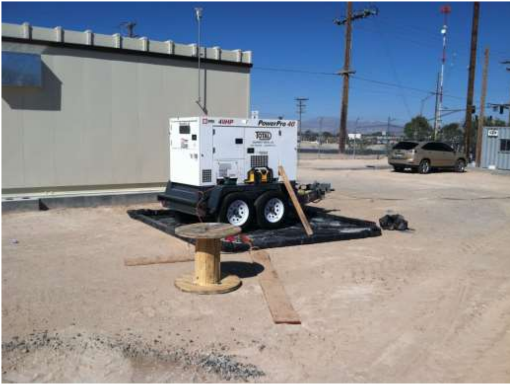
Figure 4 – Generator is equipped with secondary containment. View northeast, 03/30/15.
