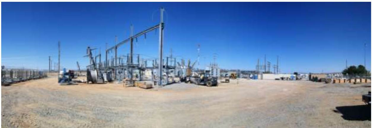
Figure 1 – Installation of the substation pad continued during the subject period. View northeast, from top: 03/17/15, 03/24/15 and 03/30/15.
