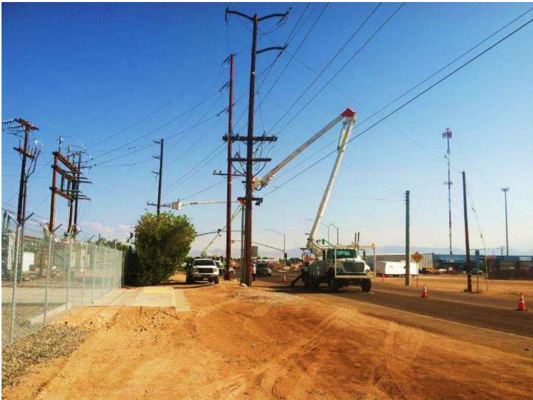
Figure 3 – Line work occurred adjacent to the Downs Substation during the subject period. View north, 04/23/15.
