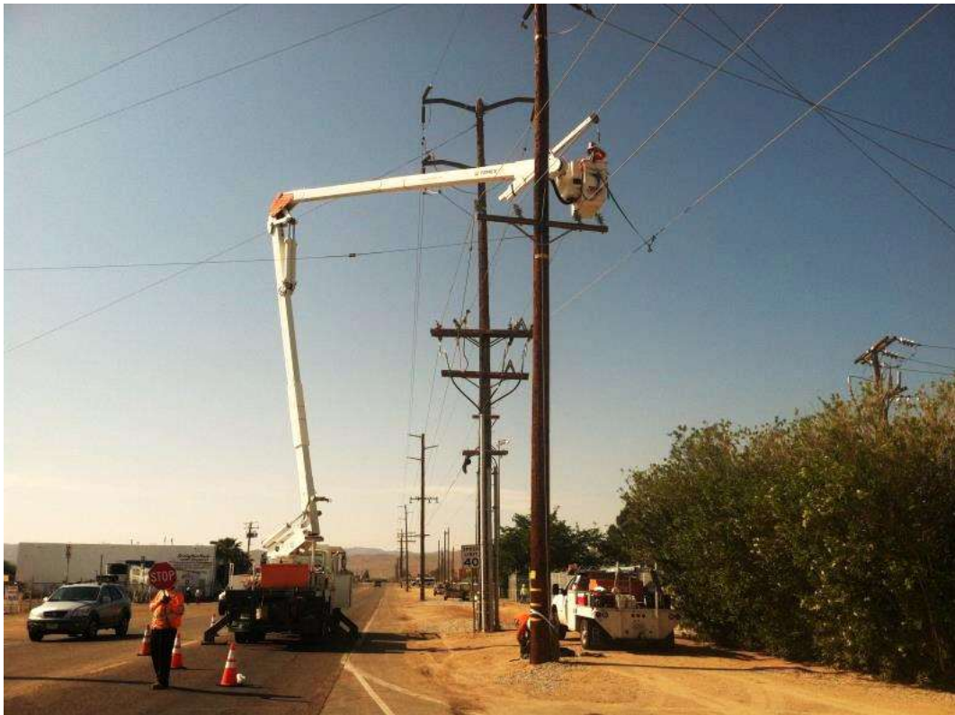
Figure 4 – Traffic control measures were implemented during overhead work adjacent to Downs Substation. View south, 4/23/15.
