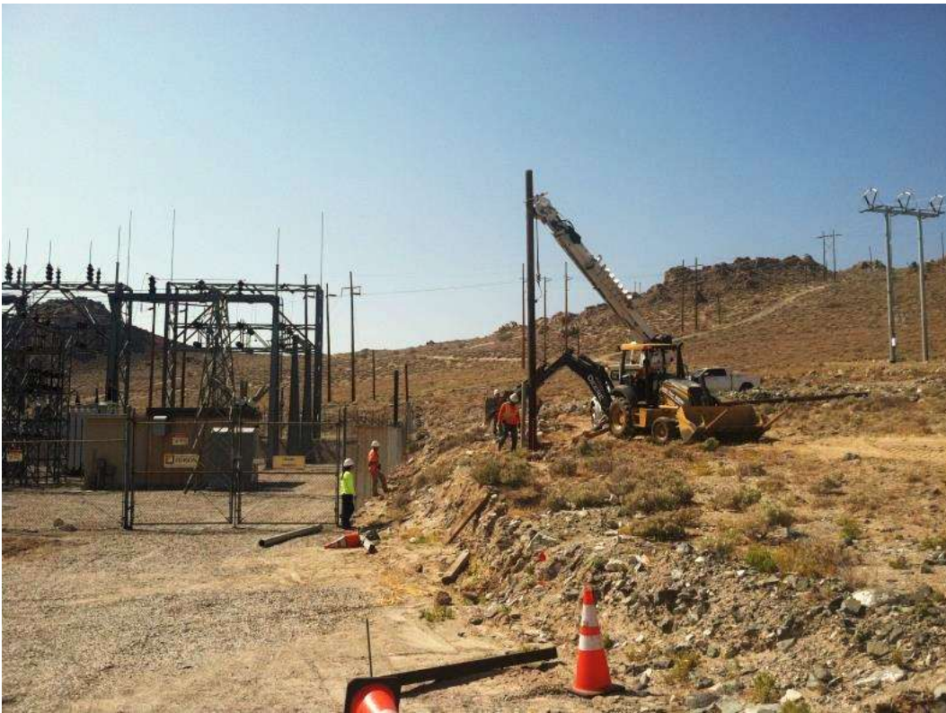
Figure 6 – Pole installation work occurred at Searles Substation during the subject period. View south, 4/23/15.
