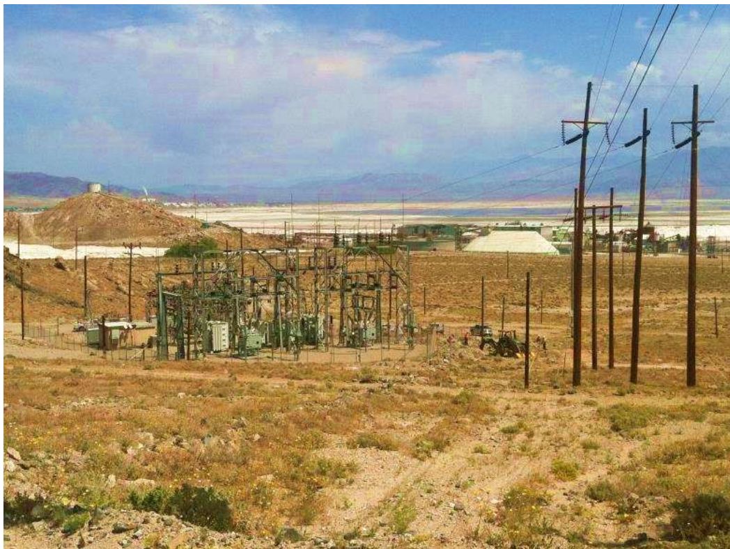
Figure 7 – Pole installation and trenching work occurred at Searles Substation during the subject period. View northeast, 4/23/15.
