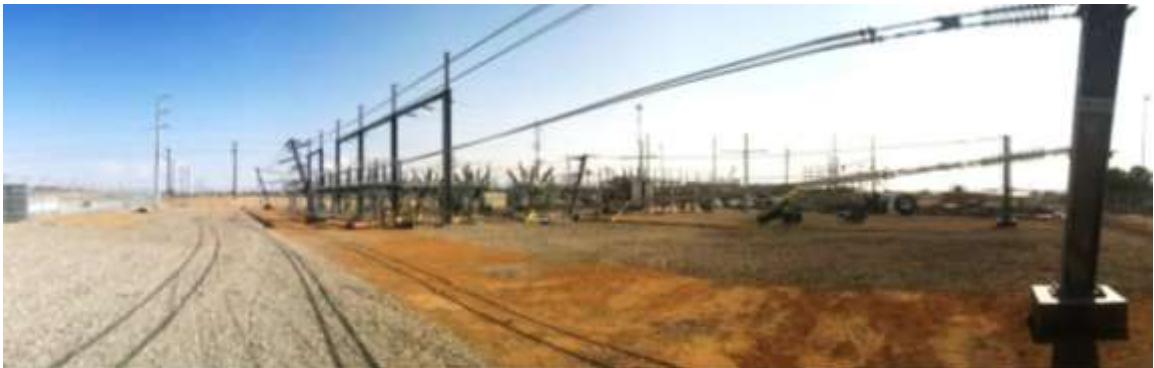
Figure 1 – Installation of the substation pad continued during the subject period. View northeast, from top: 01/27/15, 03/24/15, 03/30/15, 04/23/15.
