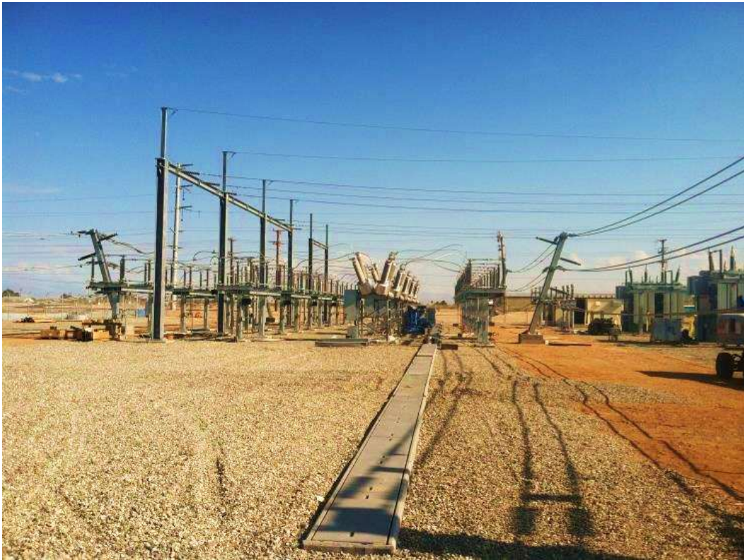
Figure 2 – Structure installation continued within the Substation expansion area during the subject period. View north, 04/23/15.
