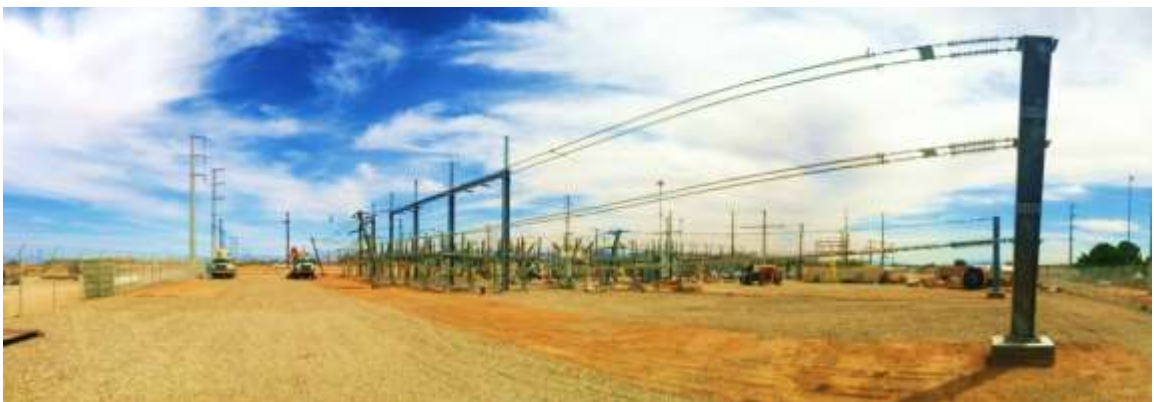
Figure 1 – Installation of the substation pad continued during the subject period. View northeast, from top: 01/27/15, 03/24/15, 04/23/15, and 04/30/15.
