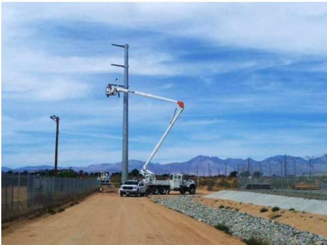
Figure 3 – Line work occurred adjacent to the Downs Substation during the subject period. View west, 04/30/15.
