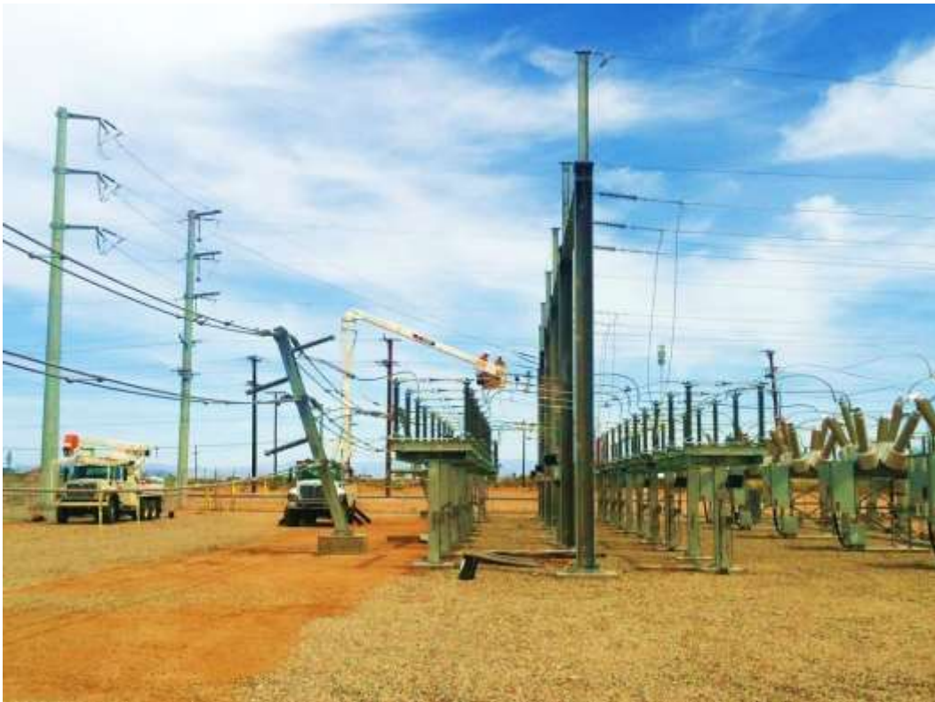
Figure 2 – Structure installation continued within the Substation expansion area during the subject period. View north, 04/30/15.
