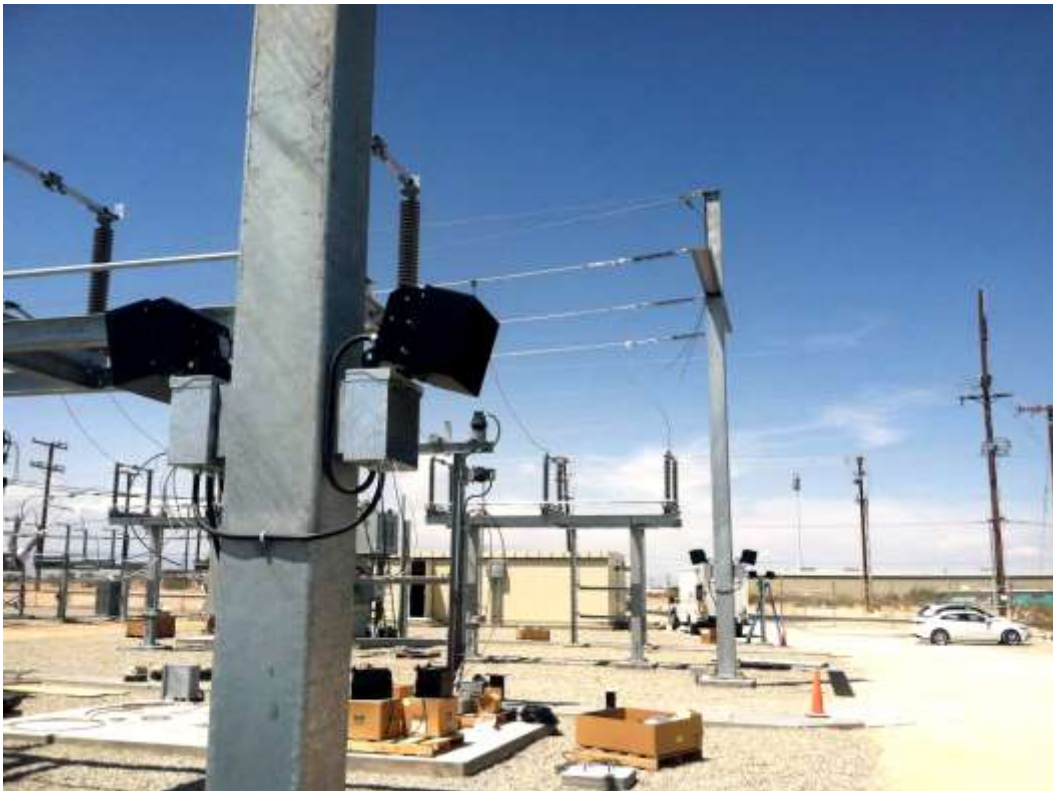
Figure 3 – Light fixtures were installed at the Downs Substation expansion area during the subject period. View North, 05/06/15.
