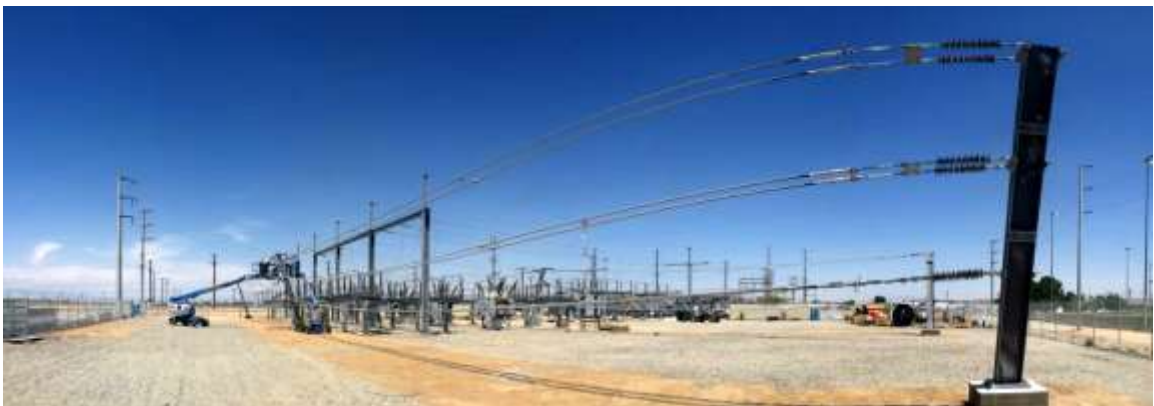
Figure 1 – Installation of the substation pad continued during the subject period. View northeast, from top: 01/27/15, 03/24/15, 04/30/15 and 05/06/15.
