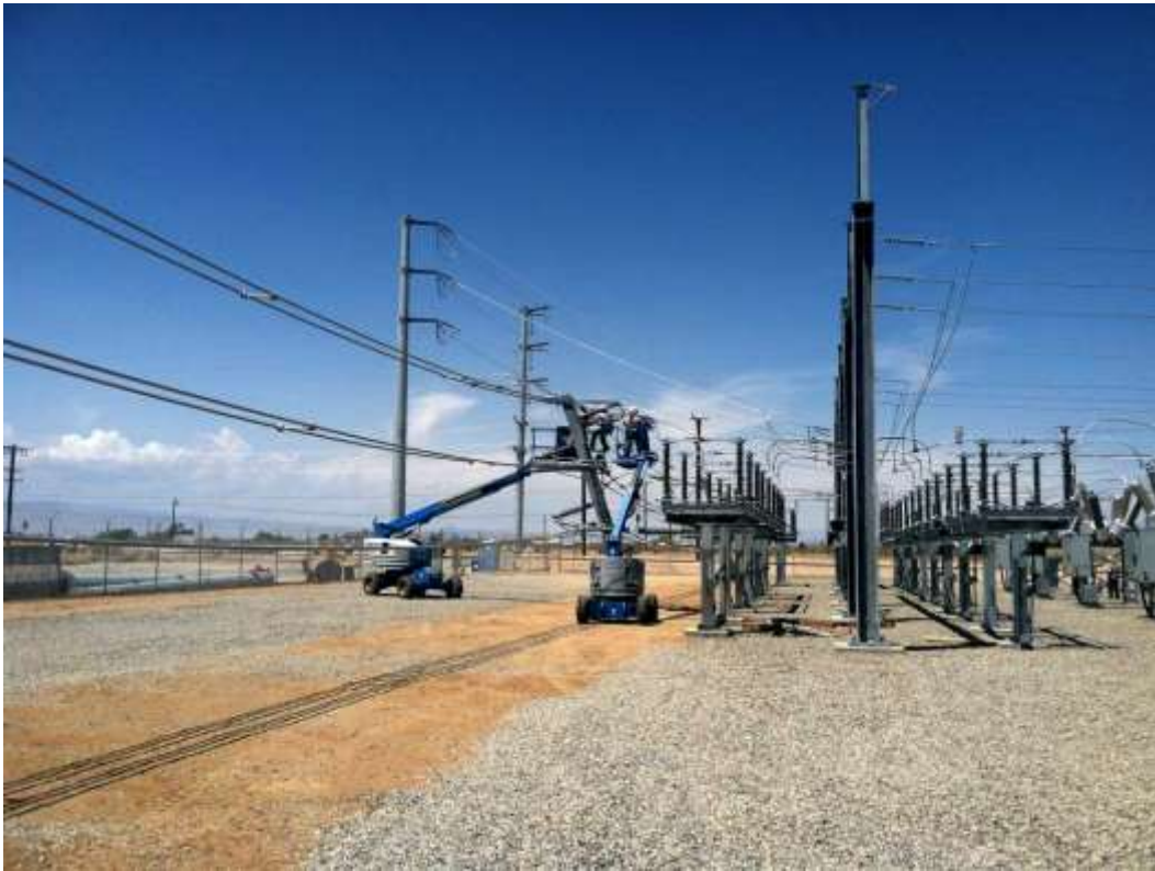
Figure 2 – Structure installation continued within the Substation expansion area during the subject period. View north, 05/06/15.
