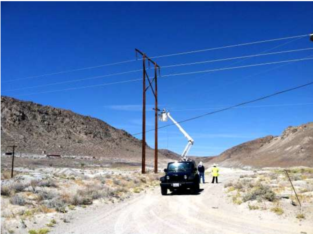
Figure 4 – Crews tighten pull rope between pole sites during the subject period. View west, 05/13/15.
