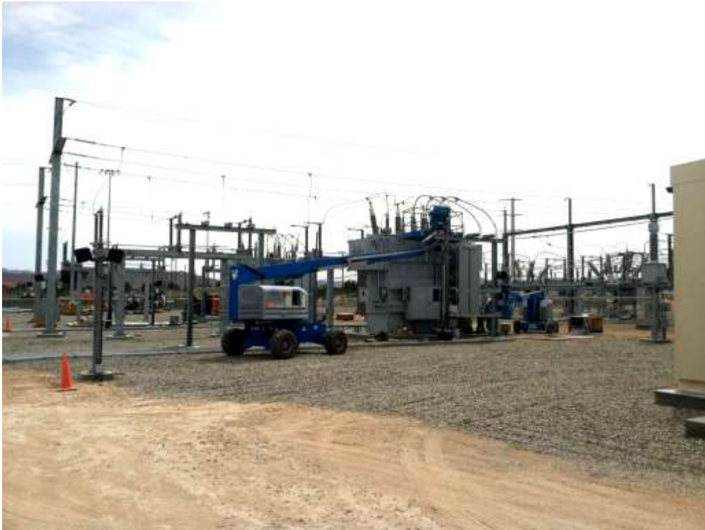
Figure 1 – Installation of the substation structures continued during the subject period. View southwest, 5/11/15.
