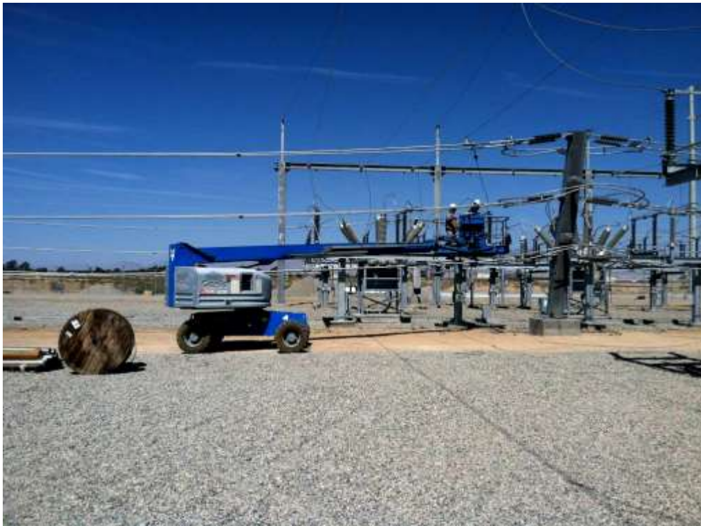
Figure 2 – Structure installation continued within the Substation expansion area during the subject period. View west, 05/13/15.
