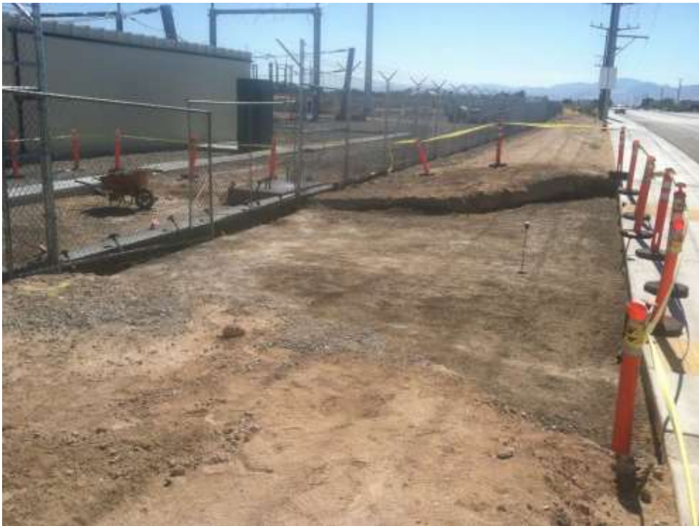
Figure 2 – Installation of a driveway apron continued during the subject period. View west, 6/16/15.
