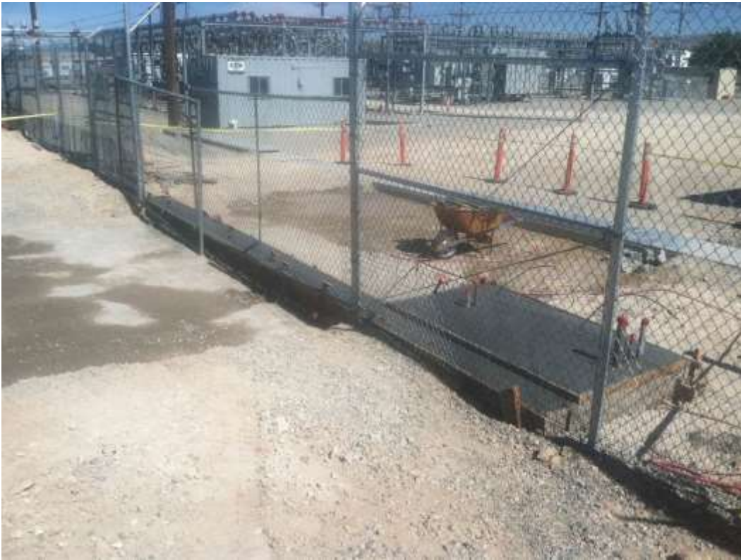
Figure 3 – Concrete installation occurred for the driveway entrance during the subject period. View southeast, 6/16/15.
