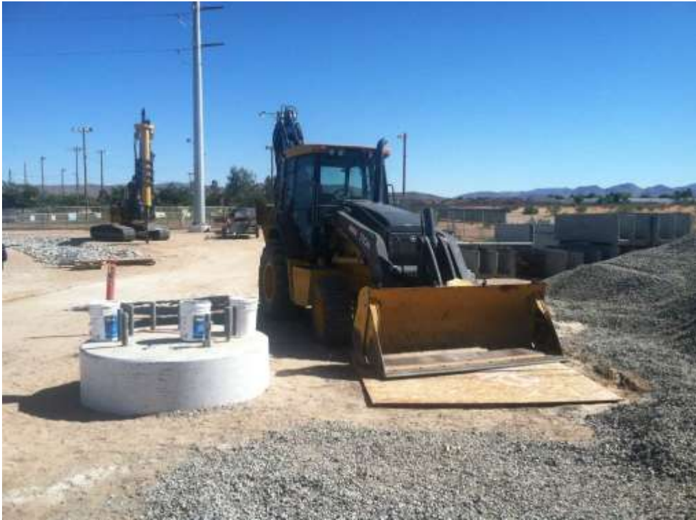
Figure 1 – Installation of new TSP foundation occurred at Downs Substation during the subject period. View south, 7/7/15.
