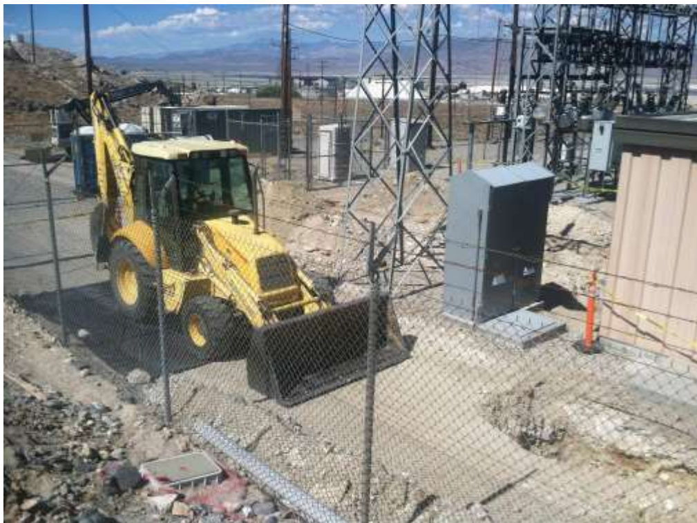
Figure 2 – Trenching and excavation work occurred at the Searles Substation during the subject period. View northeast, 7/7/2015.
