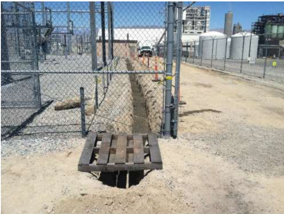
Figure 2 – Trenching work occurred at McGen Substation during the subject period. View east, 7/16/2015.
