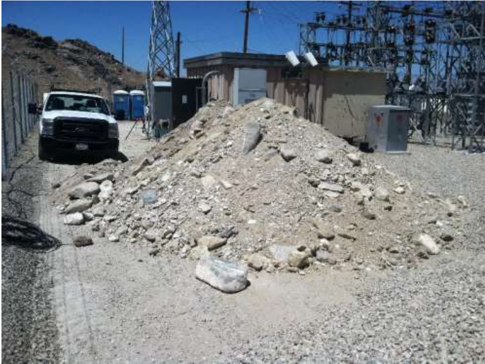
Figure 1 – Trenching and excavation work was completed at the Searles Substation during the subject period. View northeast, 7/16/2015.
