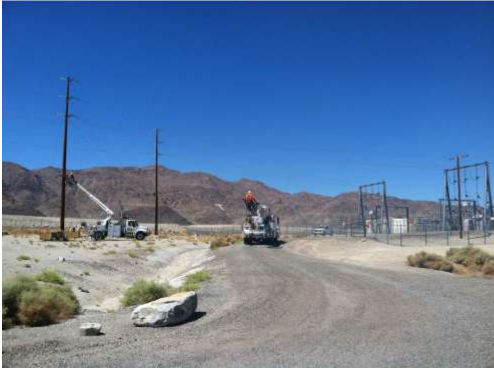
Figure 1 – Line crews installed telecom cables along the alignment between Searles and McGen (pictured) substations during the subject period. View northeast, 8/11/2015.
