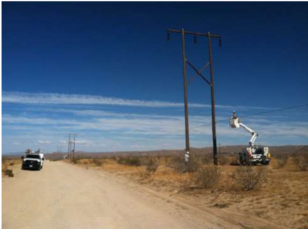
Figure 2 – Crews install telecom cables along the alignment, along West Springer Avenue during the subject period. View east, 8/11/2015.
