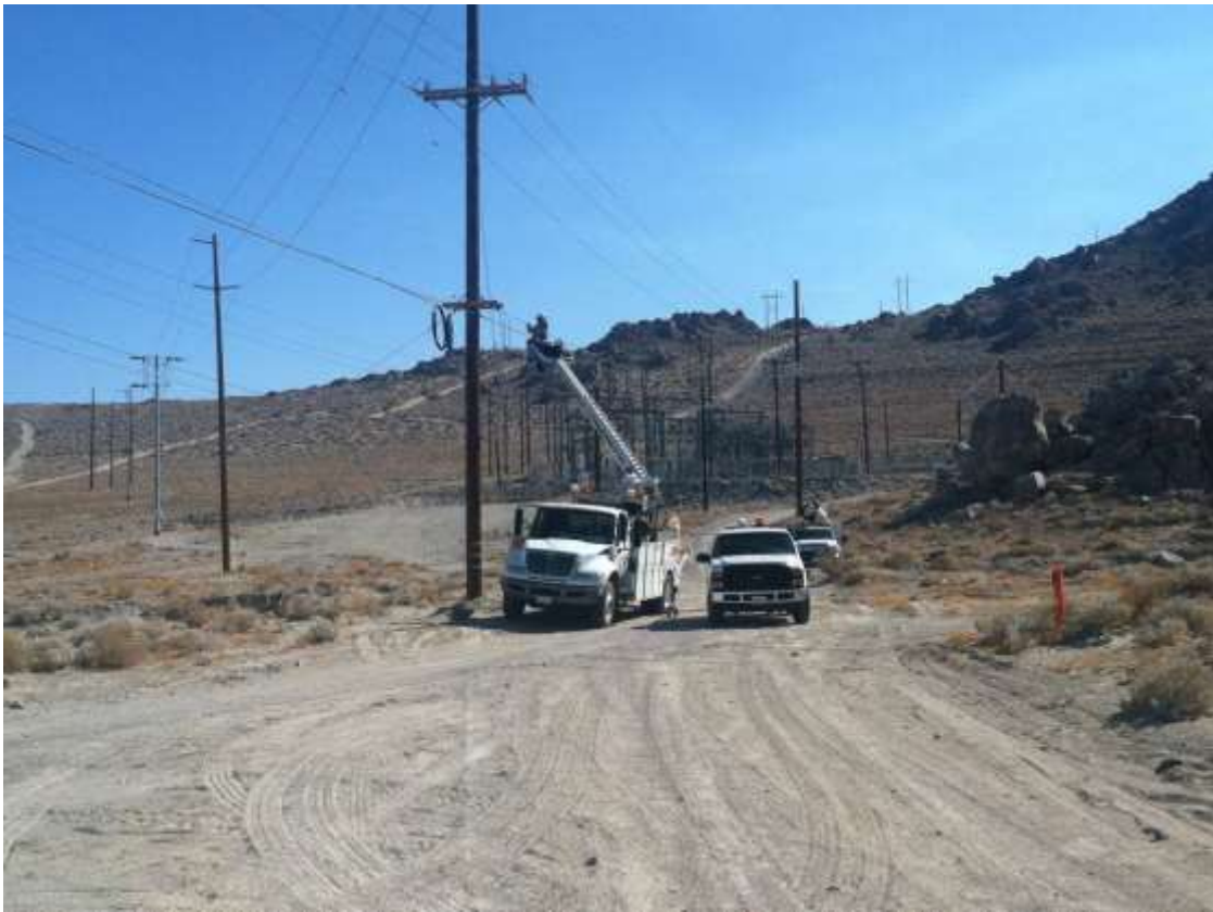
Figure 2 – Overhead crews are seen installing telecom cables along the alignment. Searles Substation is visible in the background. View south.
