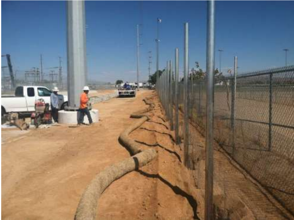
Figure 1 – Fence crews installed perimeter fencing at Downs Substation during the subject period. View east.
