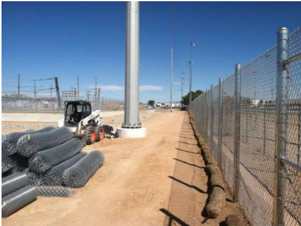
Figure 2 – Newly installed fence is seen along the southern edge of the Downs Substation area. View east.
