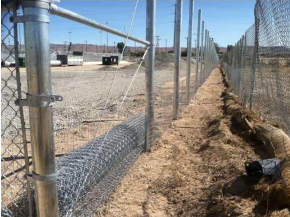
Figure 1 – Fence crews continued installing perimeter fencing at Downs Substation during the subject period. Desert tortoise mesh is seen along the bottom of the new fence line. View south.
