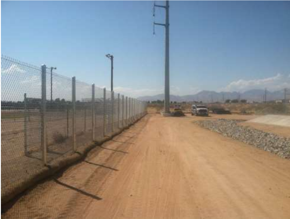
Figure 1 – Fence crews continued installing perimeter fencing at Downs Substation during the subject period. View west.
