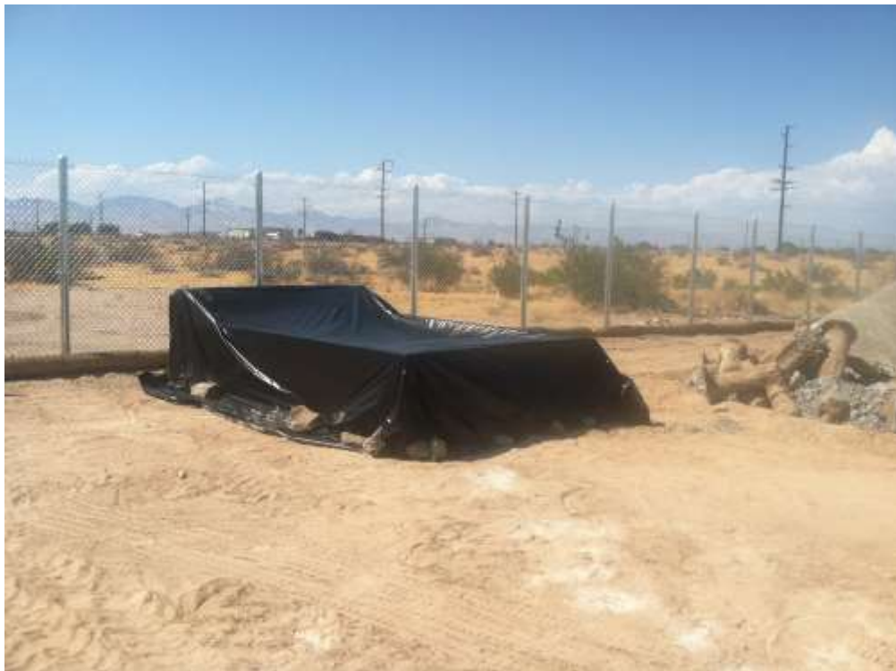
Figure 2 – The concrete washout is securely covered at the Downs Substation outer expansion area. View northwest.
