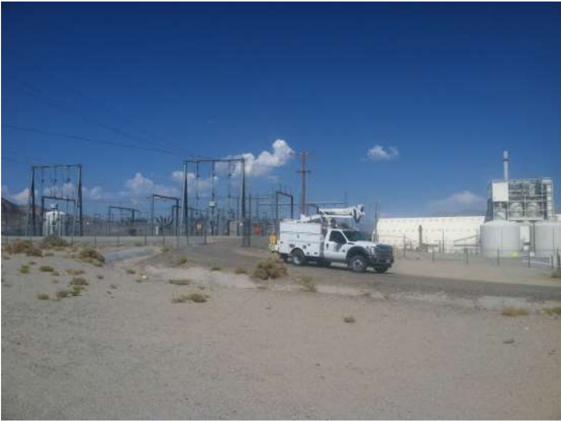
Figure 3 – Crews conducted work along the southern alignment during the subject period. View at McGen Substation, facing northeast.
