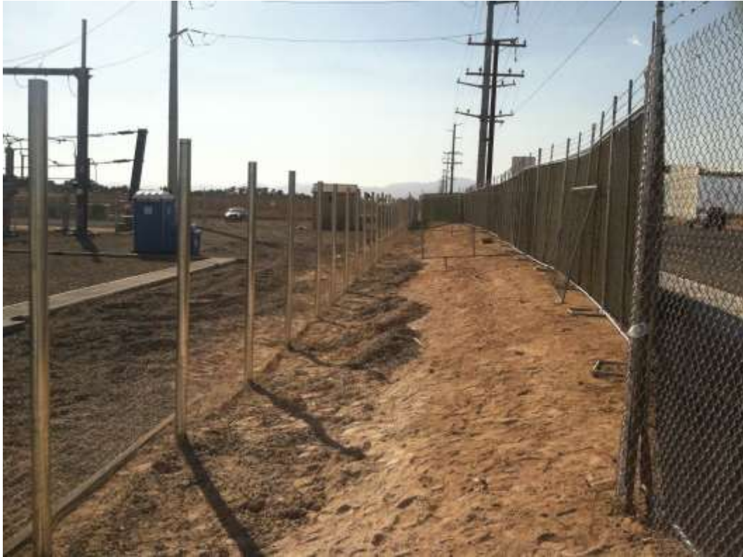
Figure 1 – Fence crews continued installing perimeter fencing at Downs Substation during the subject period. Temporary fencing is seen along the right. View west.
