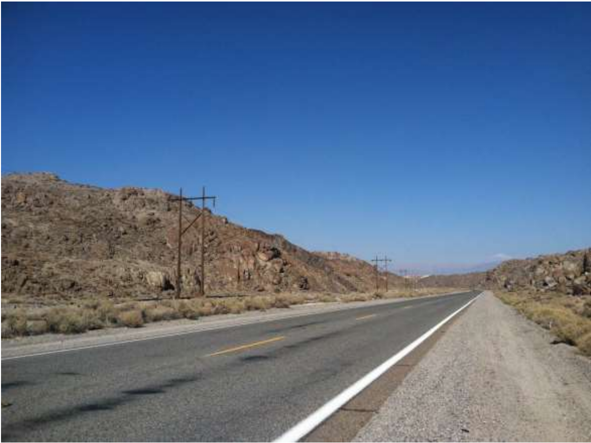
Figure 3 – Fiber line installation is nearing completion along the southern alignment (pictured). View in Poison Canyon, facing northeast.
