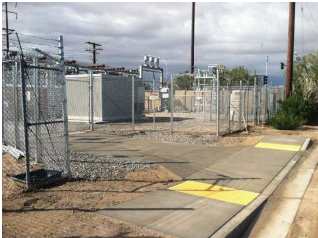
Figure 1 – Fence crews continued installing perimeter fencing at Downs Substation during the subject period. View northwest (9/29/15 above, 10/5/15 below).
