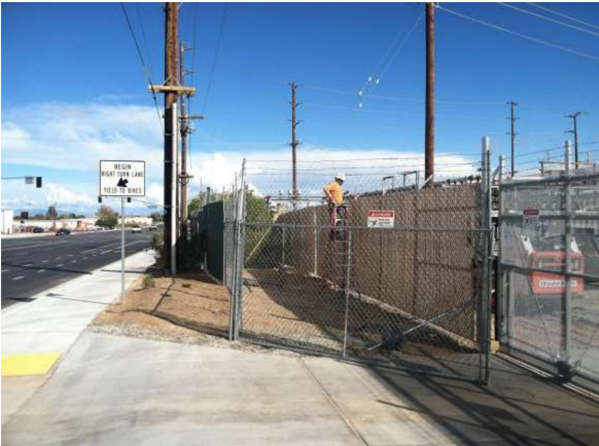
Figure 2 – Fence crews continued installing perimeter fencing at Downs Substation during the subject period. View east.
