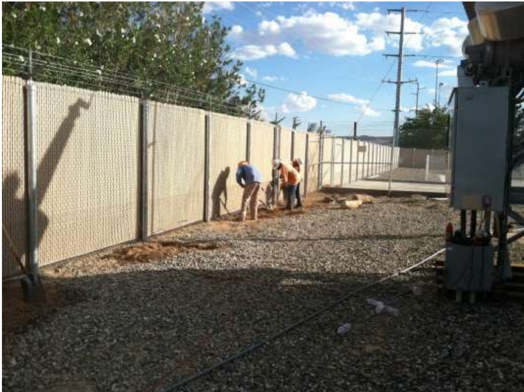
Figure 2 – Fence crews installed grounding wires along perimeter fencing at Downs Substation during the subject period. View southeast.
