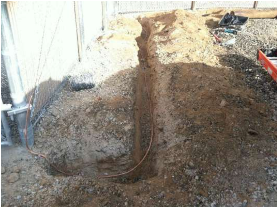
Figure 3 – Fence crews installed grounding wires along perimeter fencing at Downs Substation during the subject period. View east.
