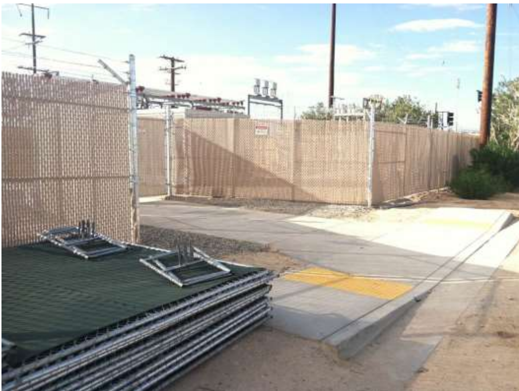
Figure 1 – Fence crews continued installing perimeter fencing at Downs Substation during the subject period. View northwest (9/29/15 above, 10/13/15 below).
