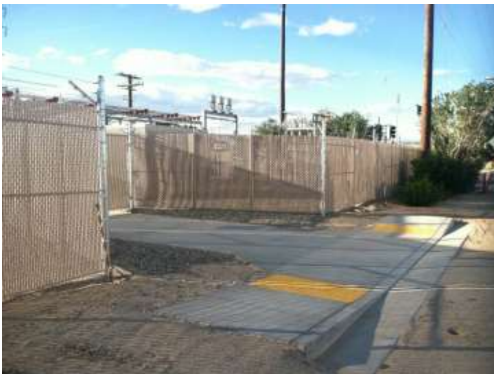
Figure 1 – Fence crews completed perimeter fencing at Downs Substation during the subject period. View northwest (9/29/15 above, 10/13/15 middle, 10/20/15 below).
