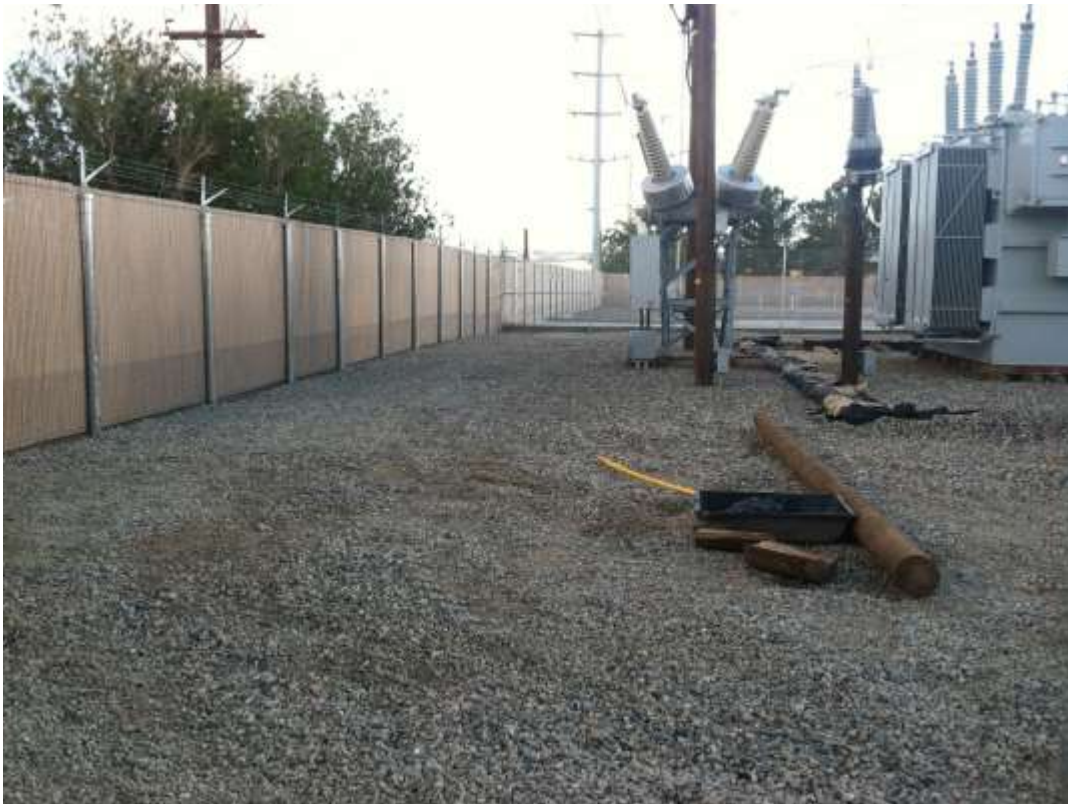
Figure 3 – Fence crews completed installing grounding wires along perimeter fencing at Downs Substation during the subject period. View southeast (10/13/15 above, 10/20/15 below).
