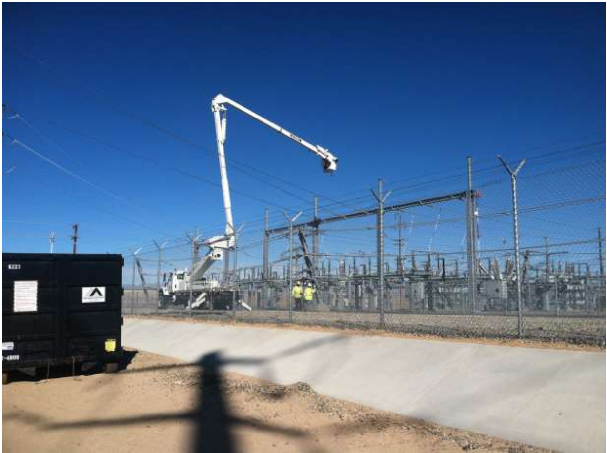
Figure 3 – Crews tied in transmission lines to the substation expansion structures during the subject period. View northeast (11/20/15).
