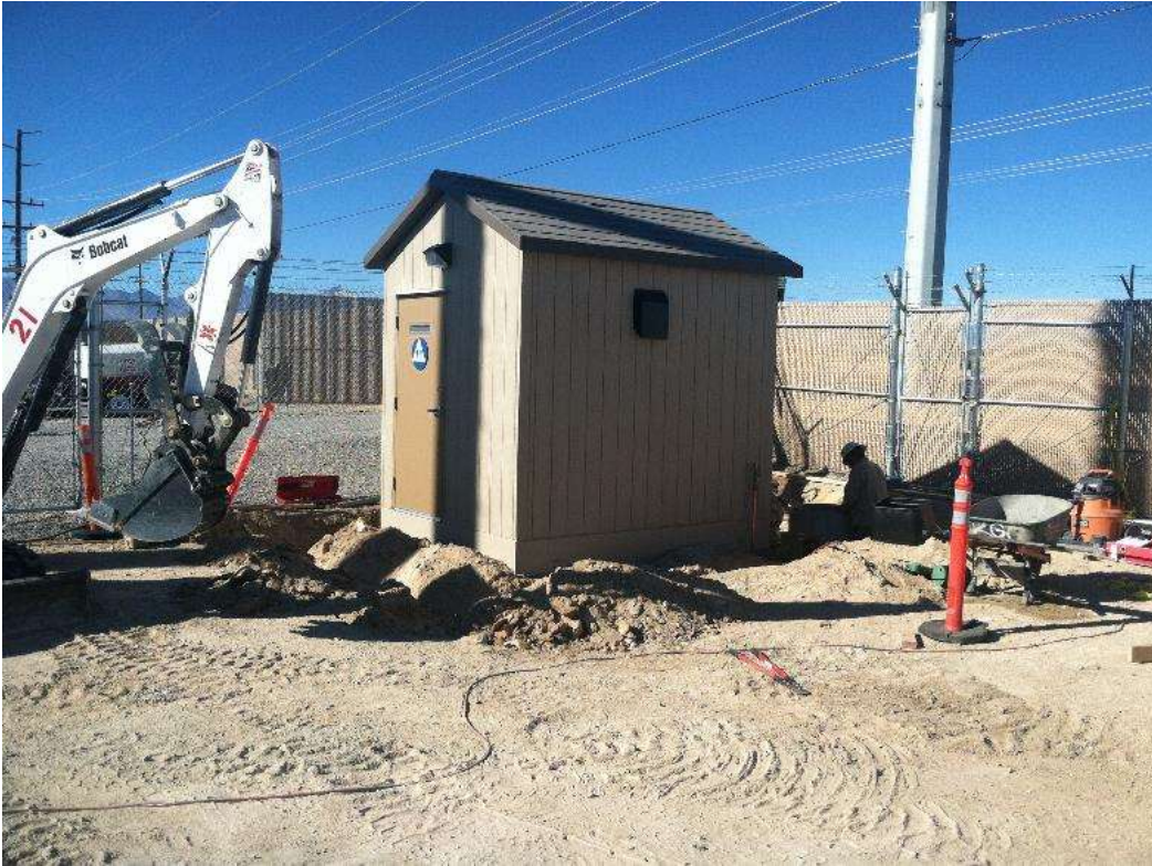
Figure 1 – Installation of a restroom facility occurred during the subject period. View northwest (11/20/15).
