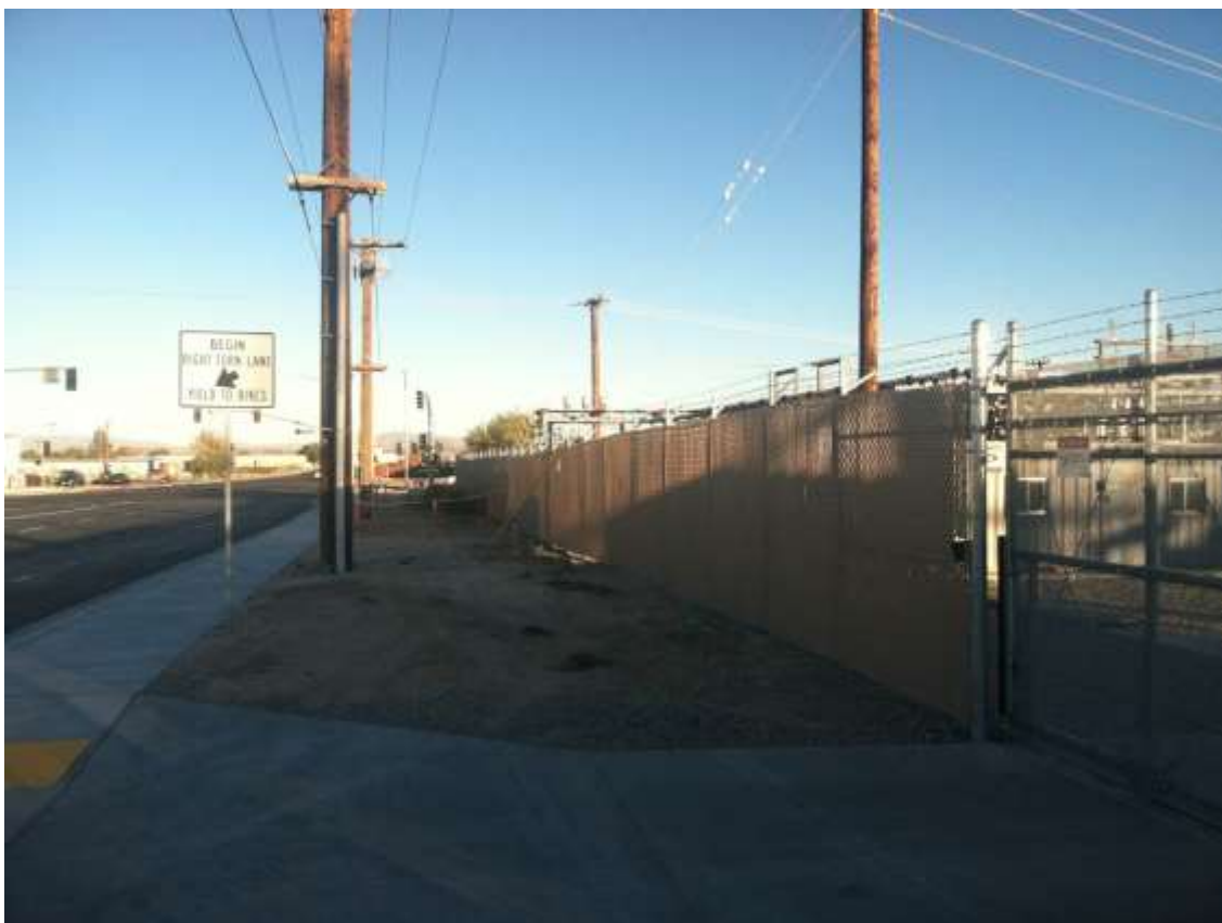
Figure 2 – Crews removed oleander bushes along the north and east boundaries of Downs Substation during the subject period. View east (10/20/15 above, 11/25/15 below).
