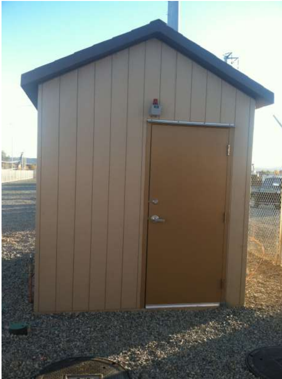
Figure 1 – Installation of a restroom facility occurred during the subject period. View south (11/20/15).
