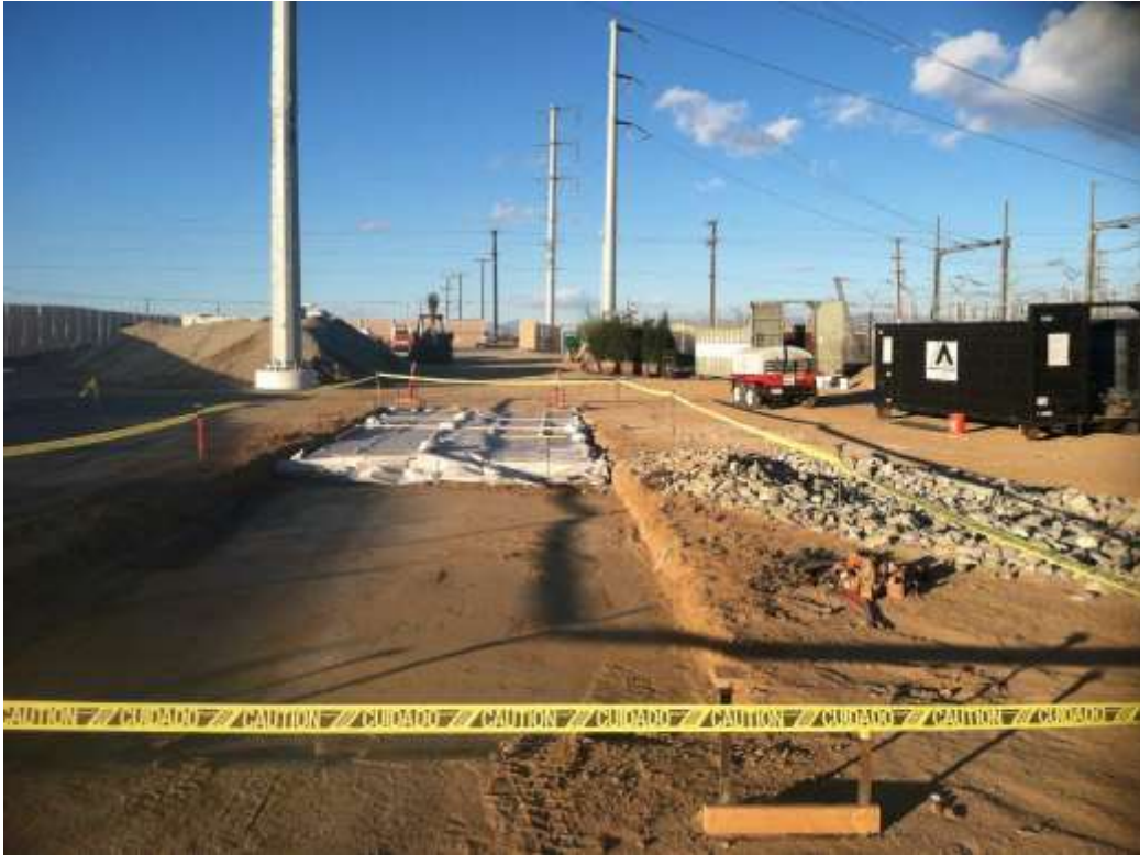
Figure 1 – Crews installed a low water crossing in the outer expansion area during the subject period. View north, 12/14/15.
