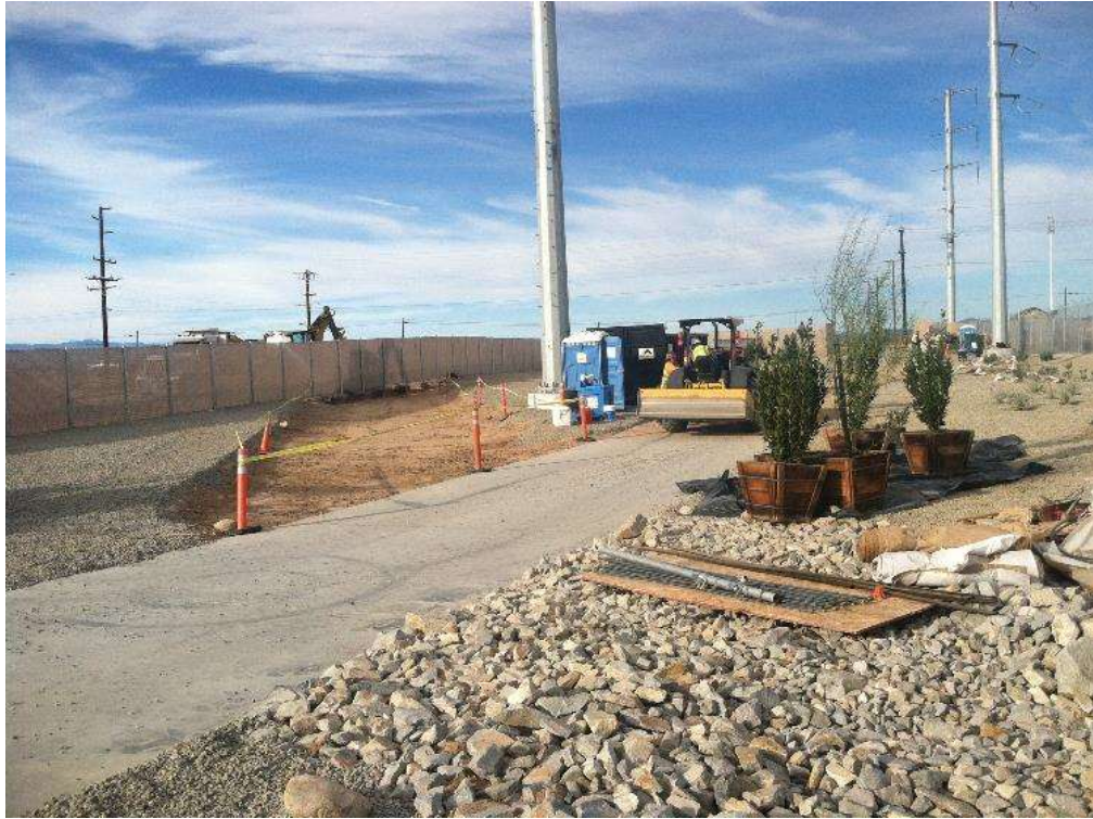
Figure 1 – Crews installed a low water crossing in the outer expansion area during the subject period. View northwest, 12/23/15.
