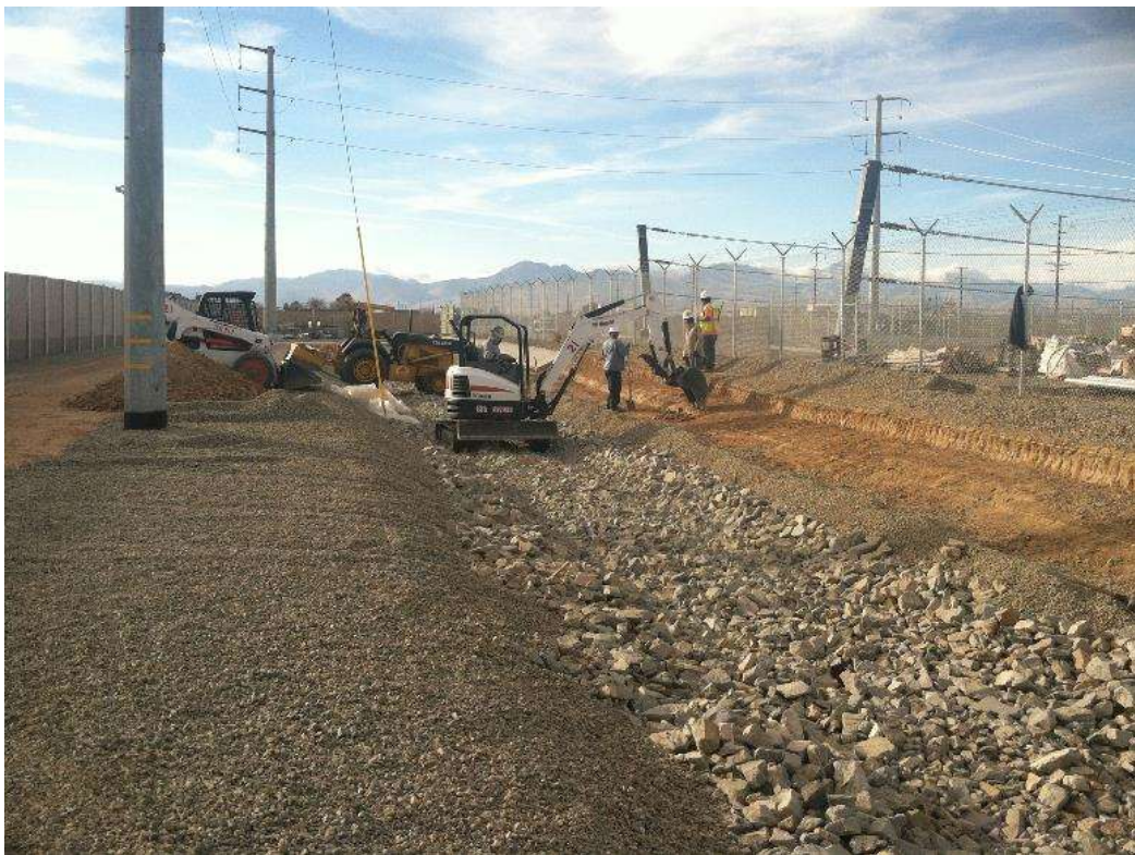
Figure 4 – Crews installed concrete along a section of the substation expansion pad perimeter. View west 12/23/15.
