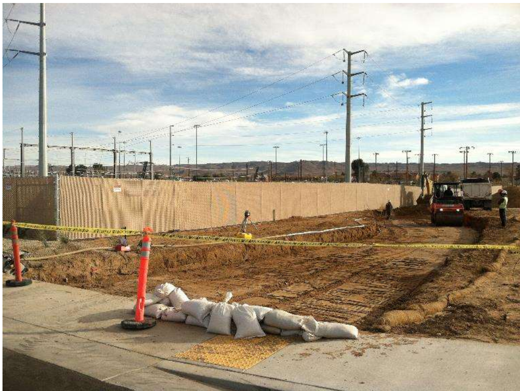
Figure 2 – Crews graded a storm water channel during the subject period. View southeast, 12/23/15.
