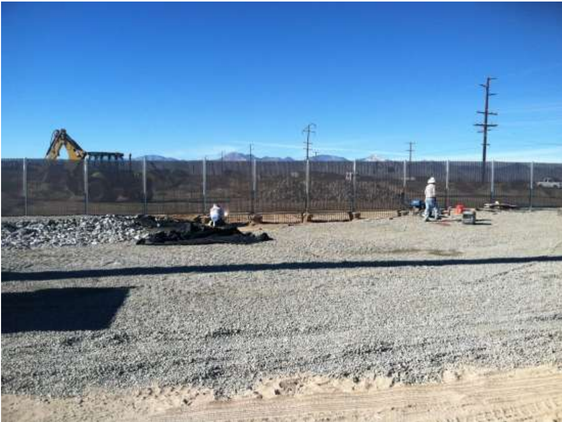
Figure 2 – Crews welded a storm water grate along a drainage corridor during the subject period. View west 12/29/15.
