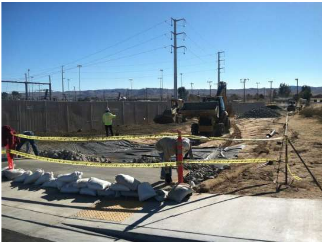
Figure 1 – Crews graded a storm water channel during the subject period. View southeast, 12/23/15 above, 12/29/15 below.
