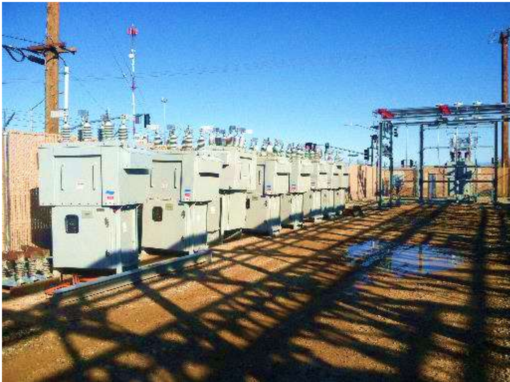
Figure 2 – New equipment for installation. View northeast 01/20/16.
