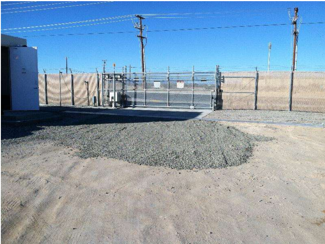
Figure 5 – Gravel apron is installed at the substation entrance to help minimize track out. View north 01/25/16.
