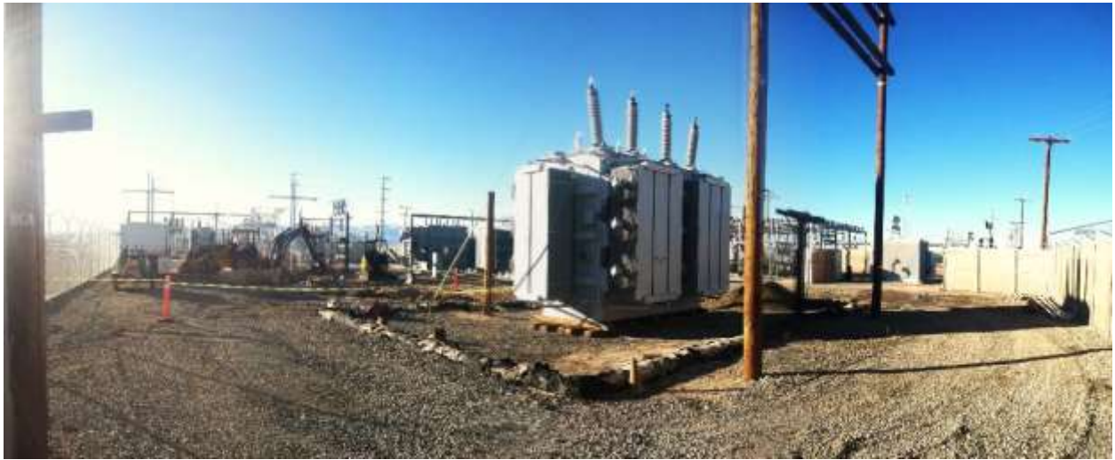
Figure 3 – Crews continued to dismantle old 33 kV structures during the subject period. View northwest 01/25/16 (above), 02/02/16 (below).
