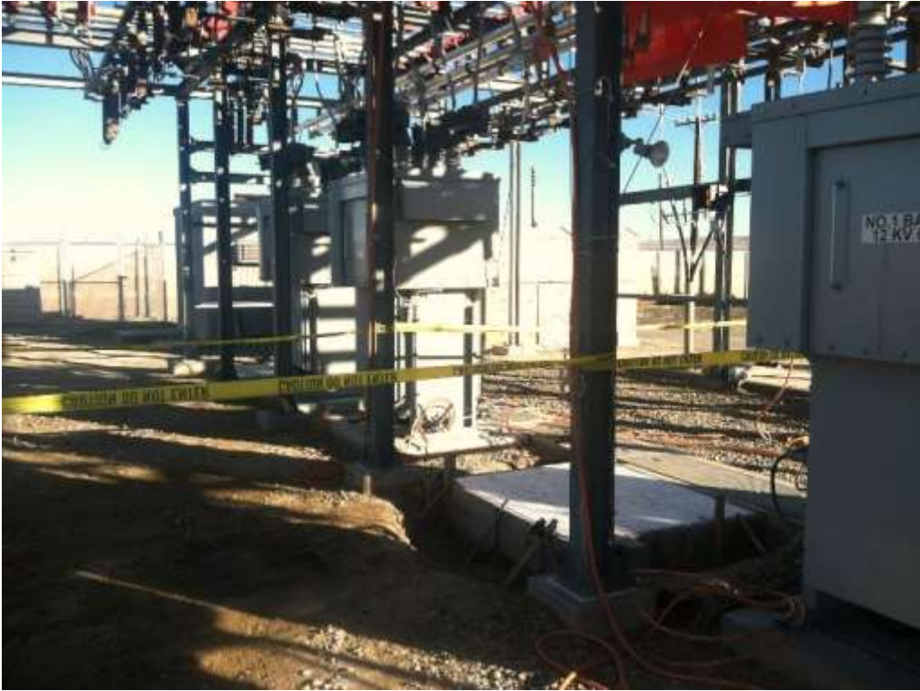
Figure 1 – Crews continued installing replacing breakers. Some new foundations were installed for these new breakers. View southeast, 02/02/16.
