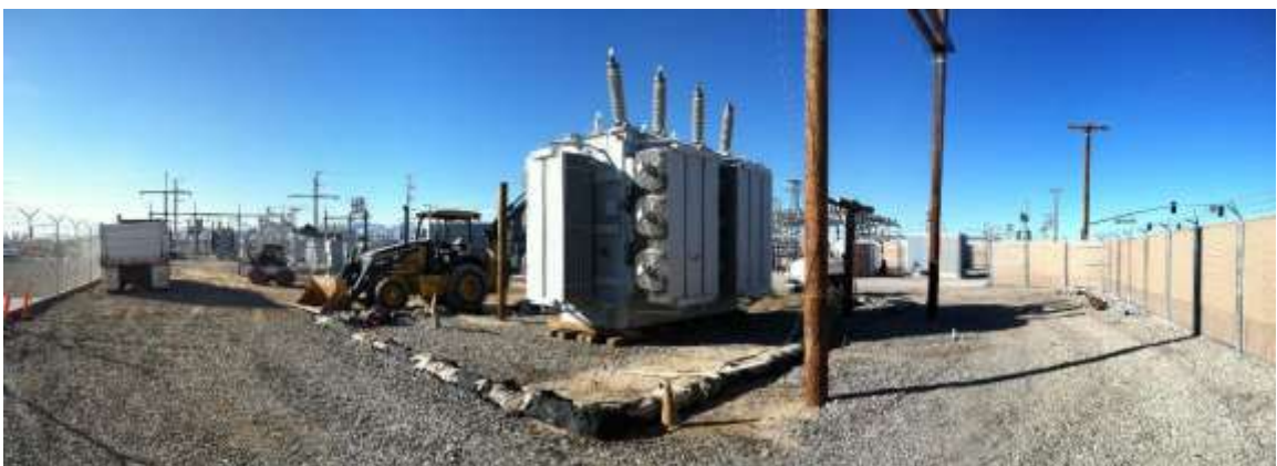
Figure 3 – Crews continued to dismantle old 33 kV structures during the subject period. View northwest 01/25/16 (above), 02/02/16 (middle), 02/08/16 (below).
