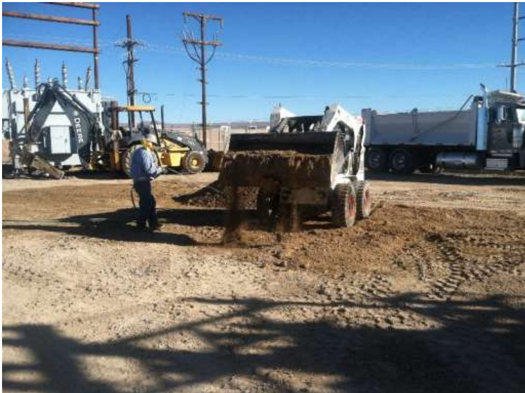
Figure 2 – Crews dismantle old 33 kV structures, removing some underground components during the subject period. View southeast 02/08/16.
