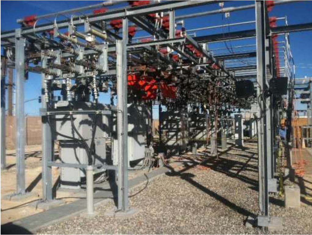
Figure 1 – Crews continued to upgrade components of the 33 kV structures during the subject period. View northeast, 02/22/16.
