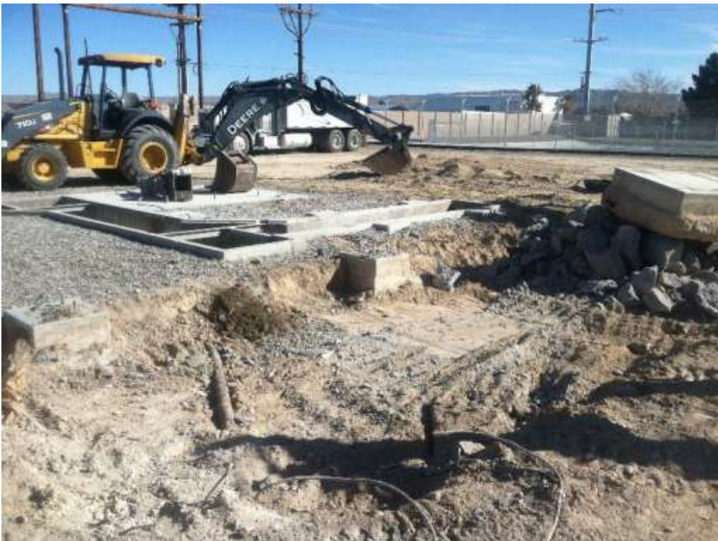
Figure 2 – Crews demolished foundations and regraded substation areas during the subject period. View southeast 02/22/16.
