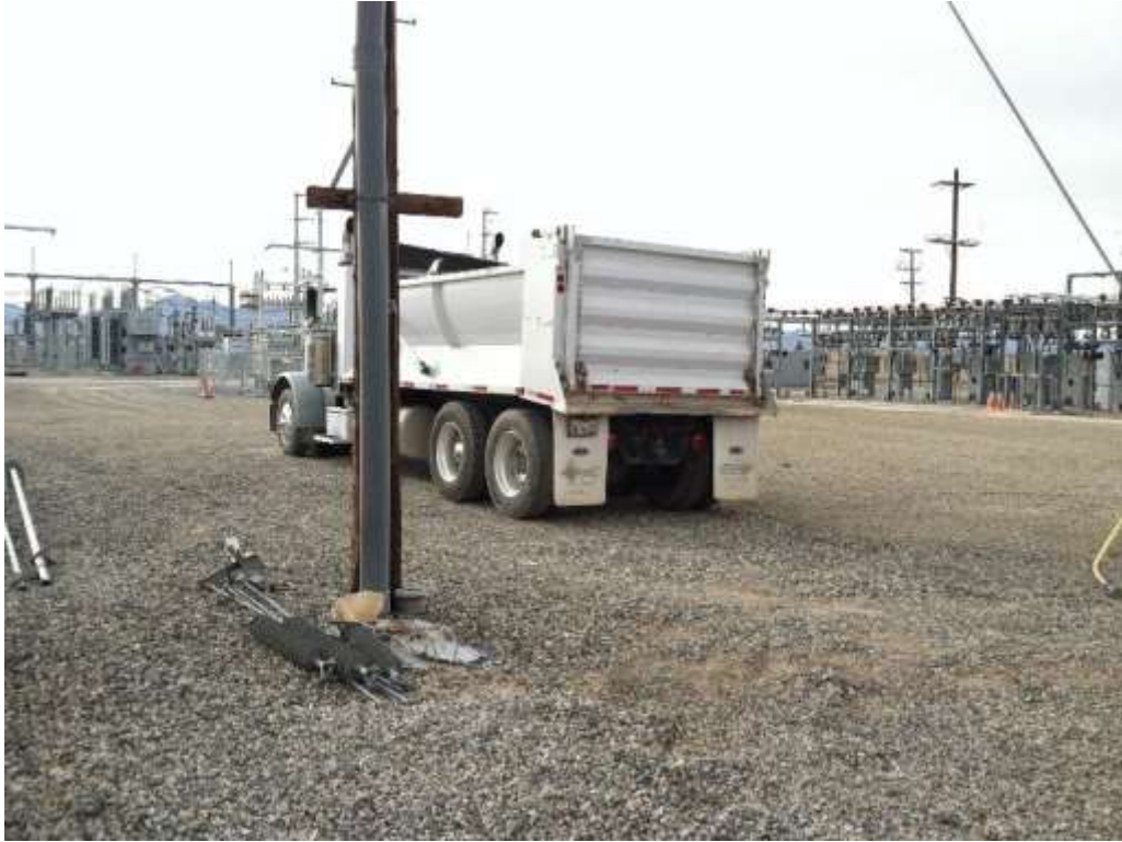
Figure 1 – Crews applied gravel to the demolition areas during the subject period. View northwest 03/03/16.
