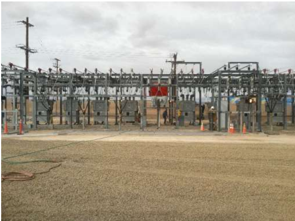
Figure 2 – Crews continued upgrading components of the old Downs Substation during the subject period. View north, 03/07/16.
