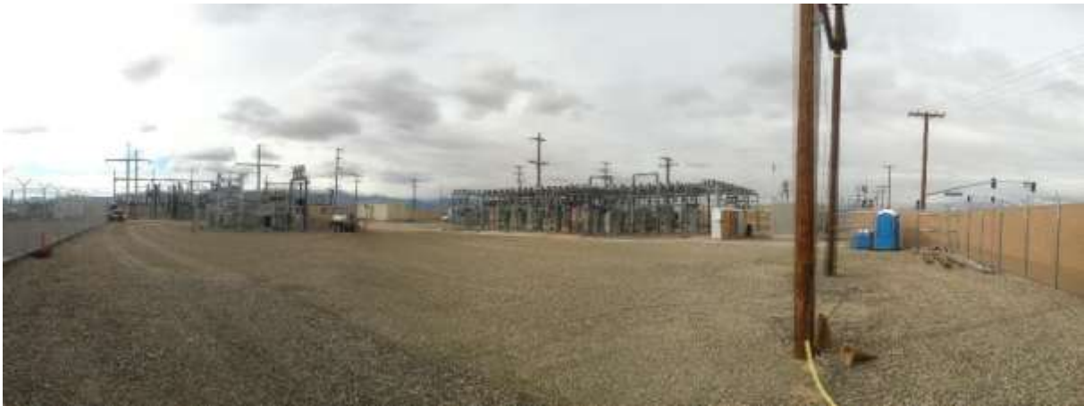
Figure 3 – Demolition work is largely complete in the old Downs Substation area. View northwest, 01/25/16 (above) 02/08/16 (middle) 03/07/16 (below).
