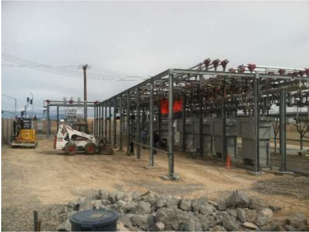
Figure 1 – Crews continued upgrading components of the old Downs Substation during the subject period. View east 03/07/16.
