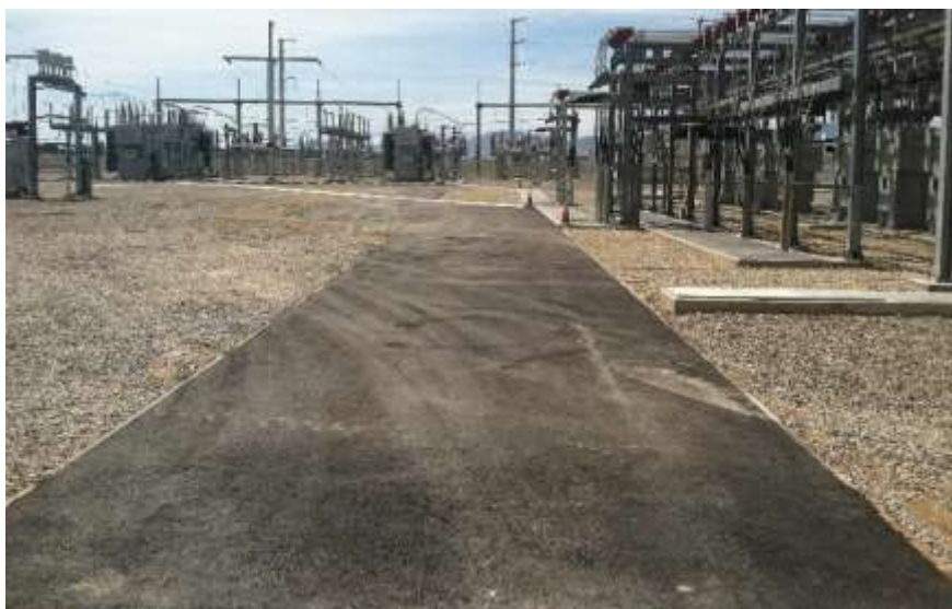
Figure 3 – Driveway renovation occurred during the subject period. View west, 4/4/16 top, 4/12/16 middle, 4/21/16 bottom.
