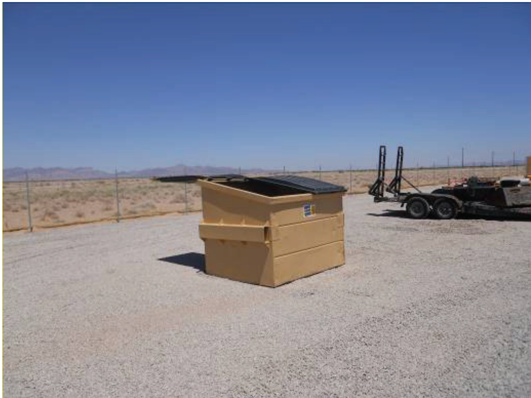
Figure 6: Trash bin left open during construction activities at the Blythe Construction Yard.
