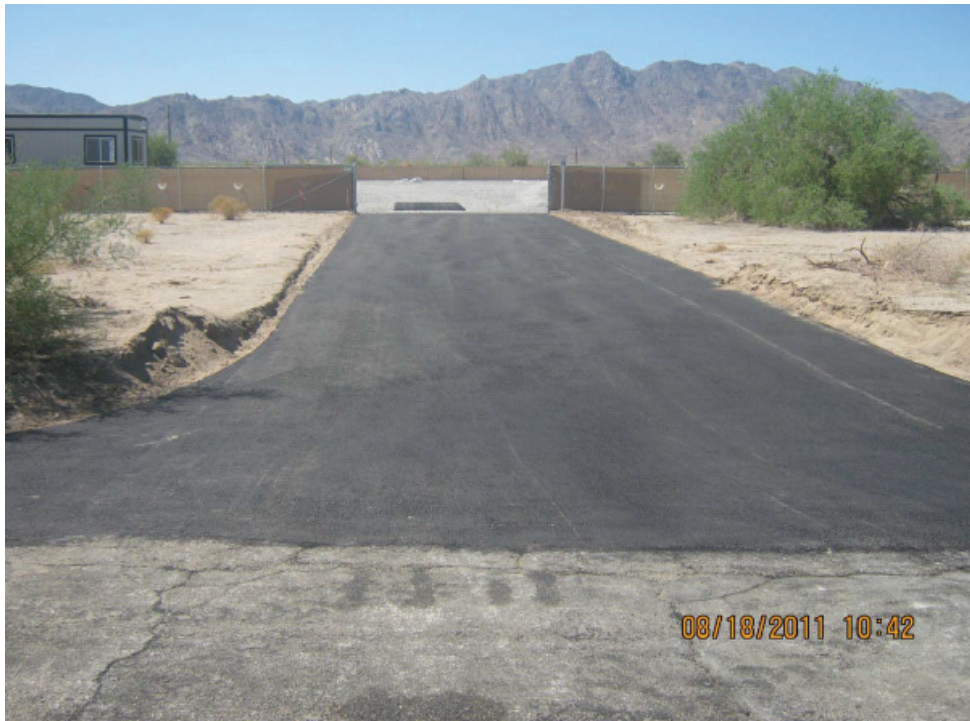
Figure 1: The ingress/egress driveways have been graded and paved at the DC2 Construction Yard.
