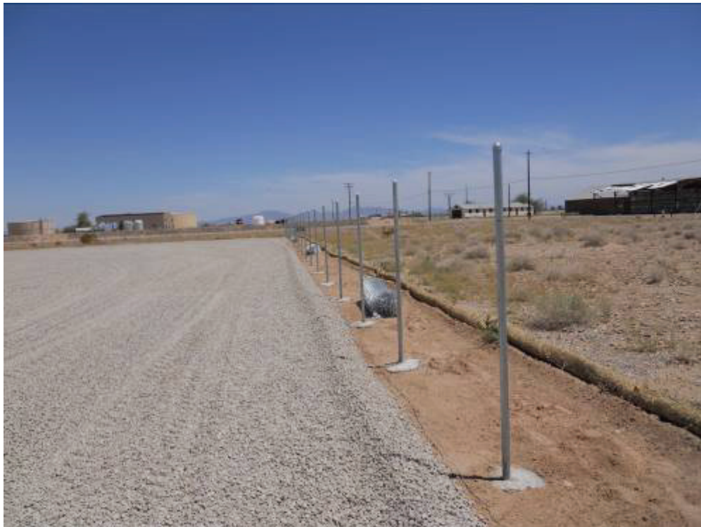
Figure 2: Construction activities at Blyth Yard included gravel placement and fence installation. View east from southern boundary.
